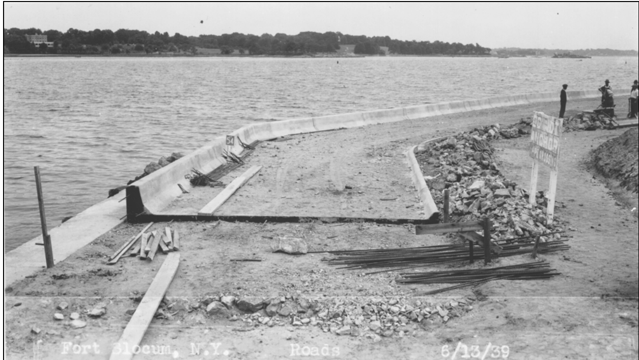
Figure 15. Construction in-progress of Parker Road at northeast corner of island, June 1939, facing northeast. In this area the road was built on fill and adjoined the seawall. View to southeast. Record Group 77, National Archives, College Park, MD.
