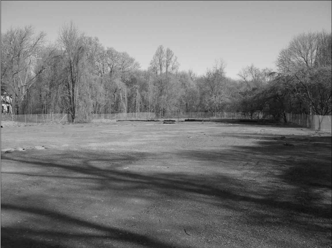
Photo 3. Southern end of Parade Ground in use as work yard (laydown area) during U.S. Army Corps of Engineers' demolition project at former Fort Slocum. Work yard has been fenced off, and the ground has been covered with geotextile fabric and gravel. Photo taken during hiatus in demolition project, April 2006. Facing north.
