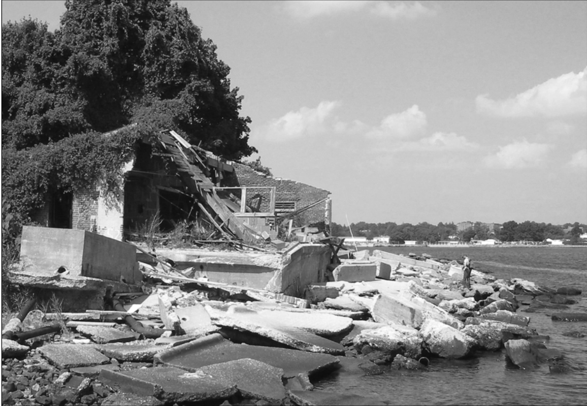
Photo 7. Seawall on northern shoreline of Davids Island (Segment F) adjacent to Sewage Tank House (Building 52, at left), facing northwest. This section of seawall is in ruinous condition, and in the center of the photograph, the wall once stood approximately at the edge of the water at right. Scattered large slabs of concrete are remnants of the collapsed pavement of Parker Road, which formerly ran between the building and the seawall.
