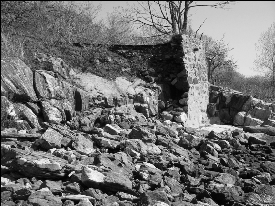
Photo 15. Seawall on southern shoreline of Davids Island (Segment K) from south of the Mortar Battery (Buildings 125-127), facing northeast. The high stone wall in this area, now collapsed, was constructed to retain the fill on which Parker Road was constructed, circa 1939.
