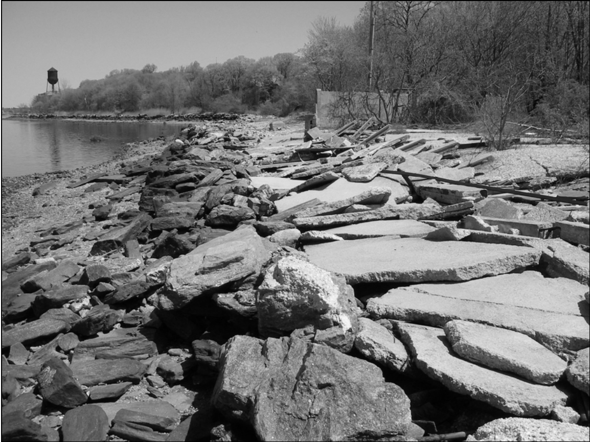
Photo 12. Seawall on western shoreline of Davids Island (Segment C), adjacent to Coal Yard (Building 27A), facing northeast. Seawall is in ruinous condition, and its location is marked by standing groups of stones along edge of gravelly beach at center left. Concrete slabs at right are from the collapsed pavement that formerly adjoined the seawall in this area and from the wall that enclosed the Coal Yard.
