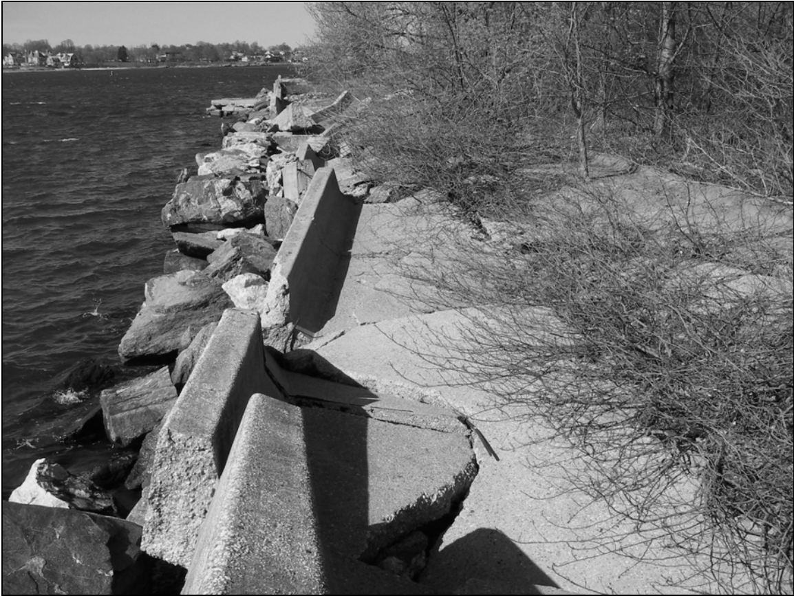
Photo 8. Seawall on western shoreline of Davids Island (Segment C) from west of Building 43, facing north. Concrete slabs are collapsed remnants of Parker Road, which was located immediately adjacent to the wall.
