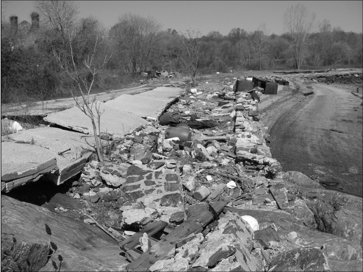
Photo 1. Seawall on eastern shoreline of Davids Island (Segment A) from east of Building 101, facing northwest. Seawall is at right along edge of beach. Upper courses of stonework have been removed by ice or waves. Concrete slabs at left belong to a collapsed section of Parker Road. Chimneys at upper left are part of Building 102.
