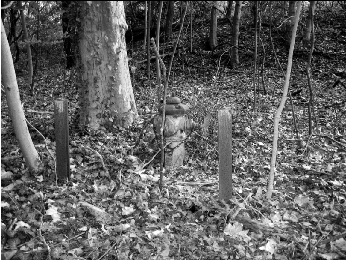
Photo 10. Fire hydrant, vicinity of Building 135, facing northeast.
