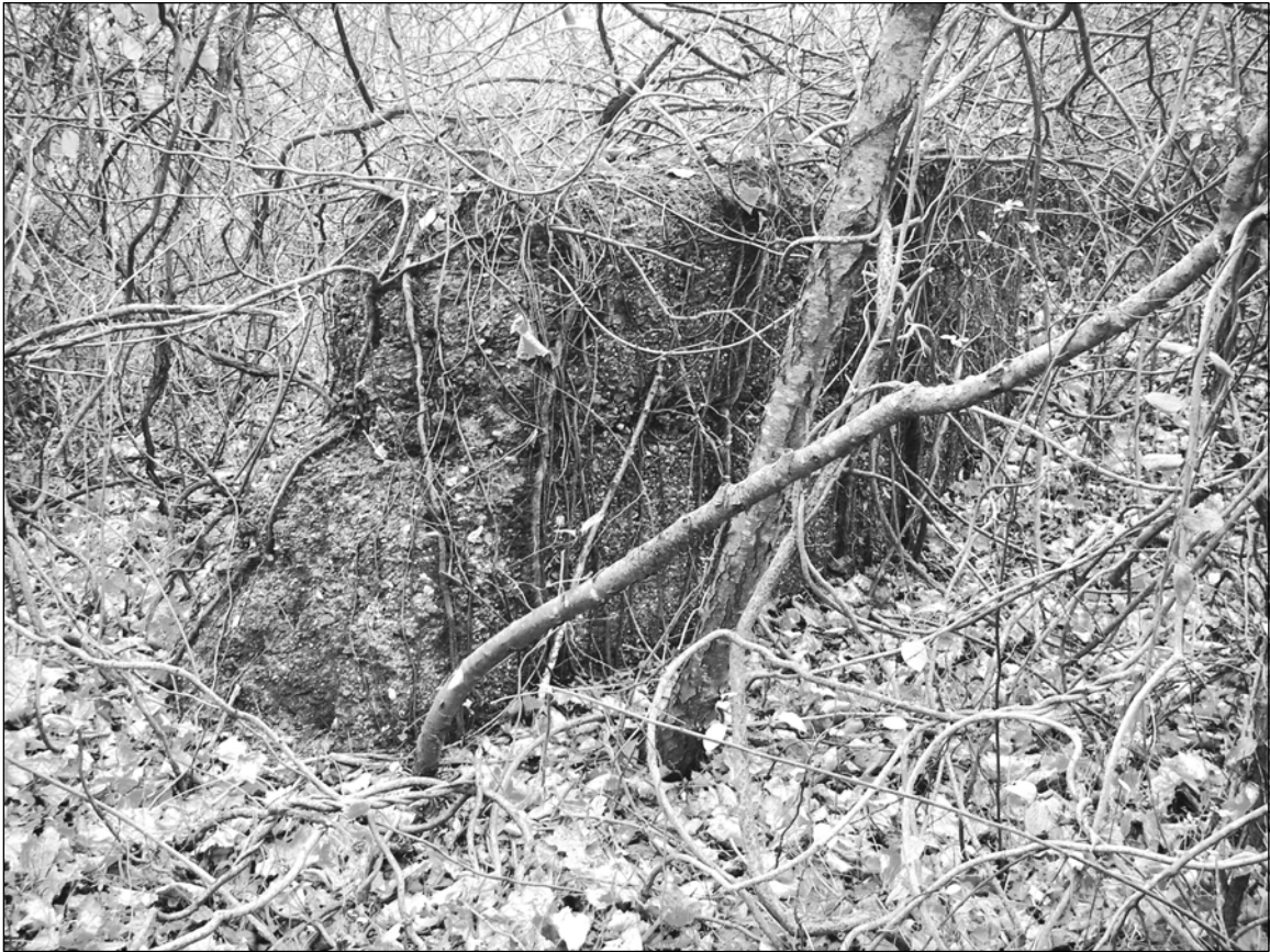
Photo 4. Limit of demolition on the north end of northern section of concrete revetment, facing southeast.
