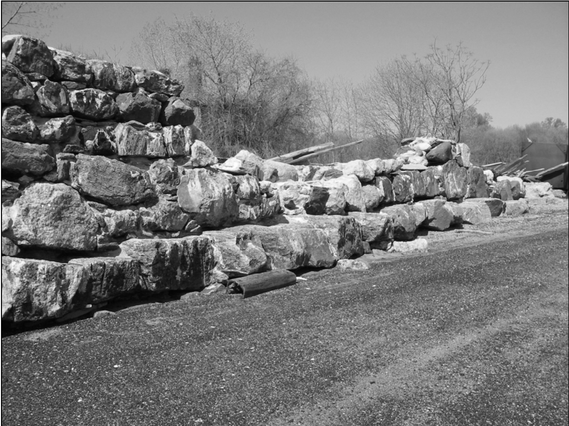
Photo 2. Eastern (seaward) face of seawall on eastern shoreline of Davids Island (Segment A) from northeast of Building 101, facing west-northwest. Chimney in background at center left behind trees is part of Building 102.
