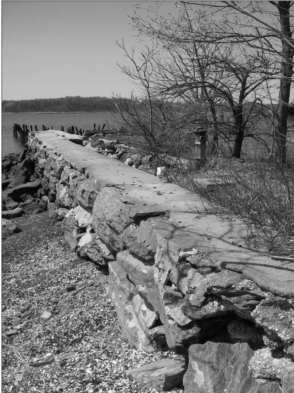
Photo 13. Seawall on southwestern shoreline of Davids Island (Segment G) from southeast of Building 30, facing west-southwest. Pilings of Passenger Dock stand in Long Island Sound beyond the end of the wall at left.
