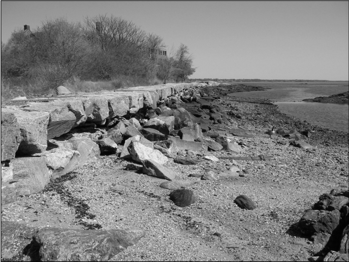
Photo 4. Eastern (seaward) face of seawall on eastern shoreline of Davids Island (Segment A) from east of Building 79, facing north-northwest. Building 60 is visible in background at left.
