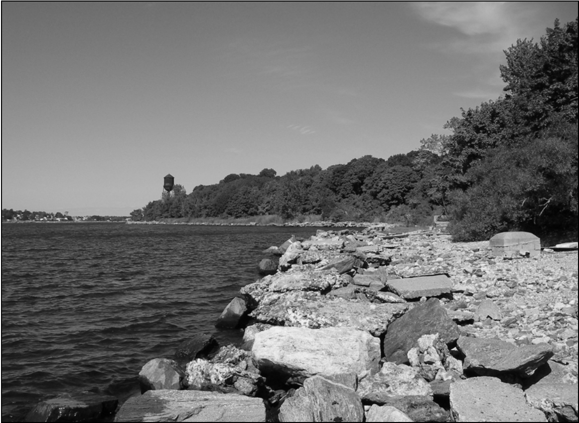
Photo 10. Seawall on western shoreline of Davids Island (Segment C) at low tide from northwest of Building 32B, facing northeast. Photographer stands atop former seawall, now in ruinous condition. Water Tower (Building 45) is visible in background at center left.
