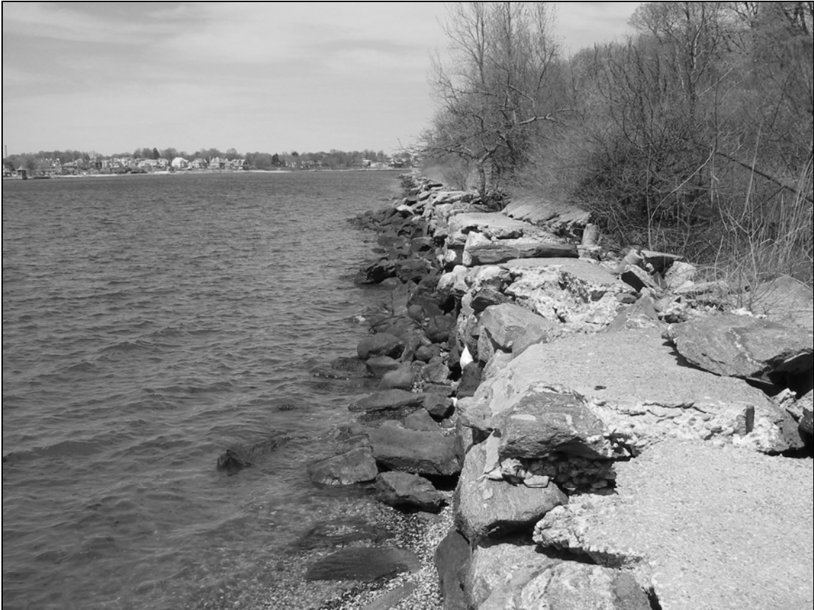
Photo 9. Seawall on western shoreline of Davids Island (Segment C) from west of Building 9, facing north. The Officers' Tennis Courts are situated in the brush at the right edge of the photograph.
