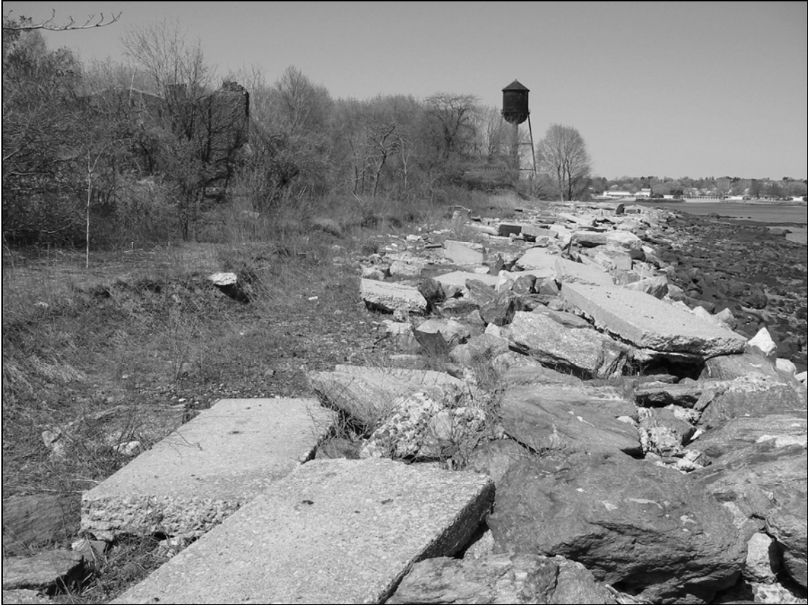
Photo 6. Seawall on northeastern shoreline of Davids Island (Segment D in foreground) from east of Building 57, facing west-northwest. This section of seawall is in ruinous condition, and the wall originally stood along the edge of the rocky beach at right. Concrete slabs in foreground formerly formed a cap atop the wall. Erosion has cut a notch in the bank at left. Building 57 is visible in brush at upper left; the Water Tower (Building 45) stands in background at center right.
