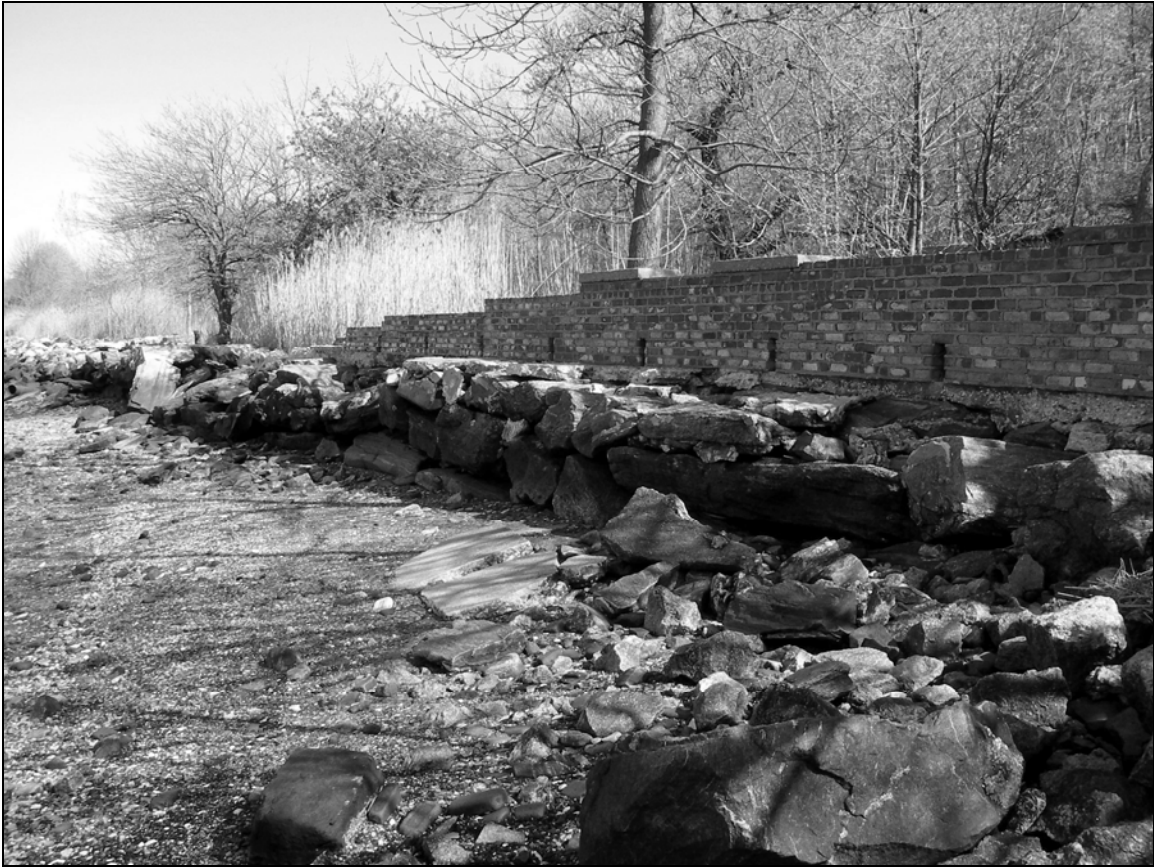
Photo 14. Seawall on southwestern shoreline of Davids Island (Segment G) from southwest of Building 131, facing north. The brick wall atop the seawall is a later addition and was probably intended as a vehicle barrier for Parker Road, which is located just behind it.
