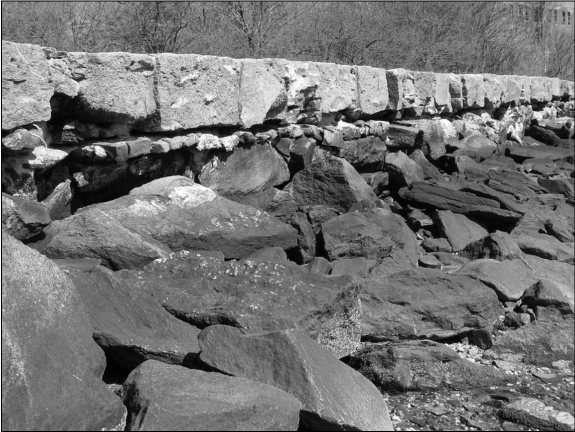
Photo 5. Detail of eastern (seaward) face of seawall on eastern shoreline of Davids Island (Segment A) from east of Building 79, facing northwest.
