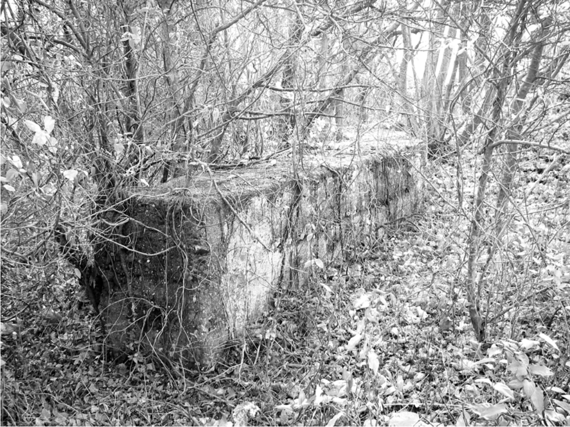
Photo 5. North end of southern section of concrete revetment, facing southeast. Note squared, finished end of wall section at left and seam line marking separate pours of concrete during construction on face of wall at center right.
