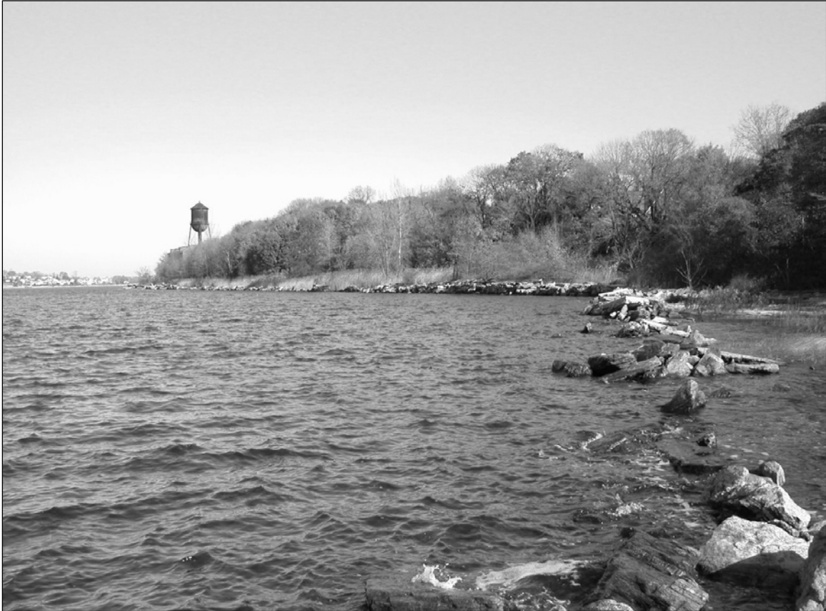
Photo 11. Seawall on western shoreline of Davids Island (Segment C) at high tide from west of Building 35, facing northeast. Remnant of seawall, now in ruinous condition, is marked by line of stones surrounded by water at right. Water Tower (Building 45) is visible in background at center left.
