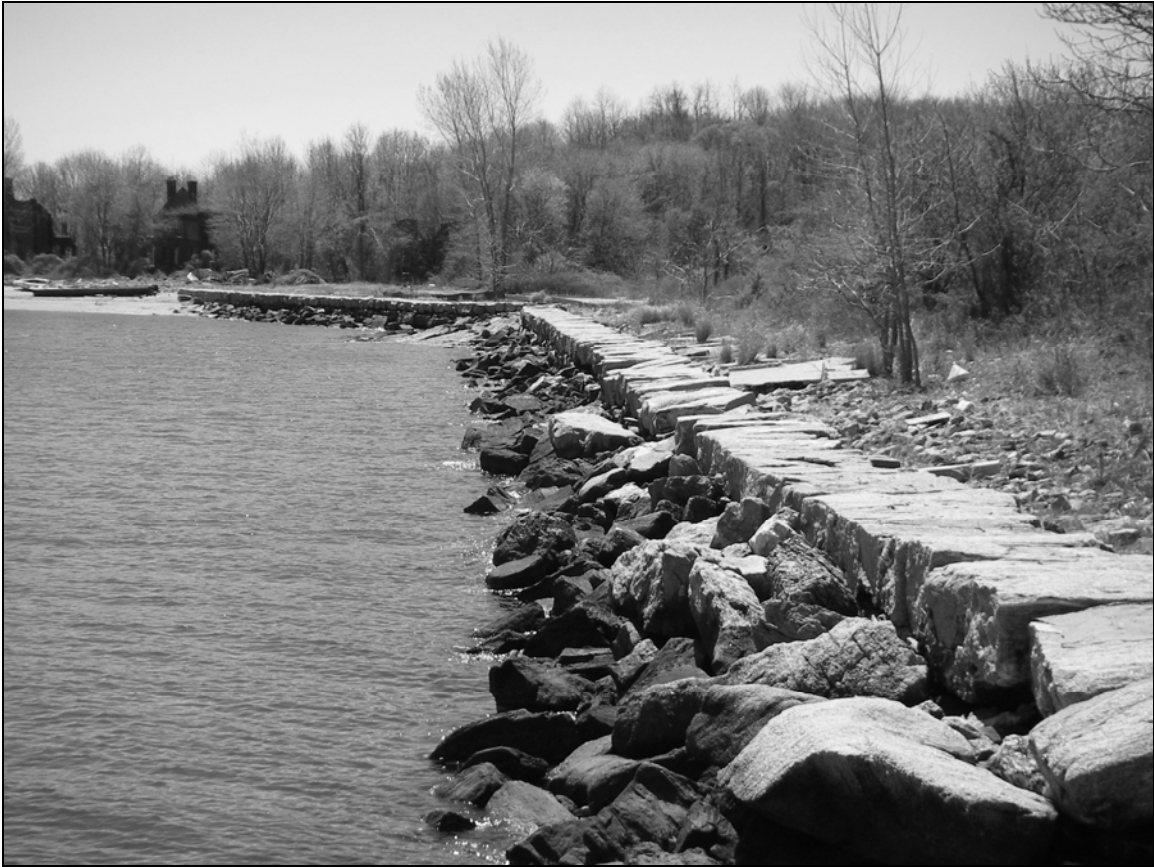
Photo 3. Seawall on eastern shoreline of Davids Island (Segment A) from southeast of Building 60, facing south.
