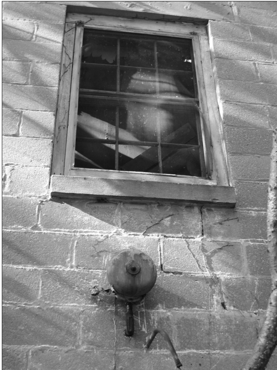
Photo 2. Southeastern façade, details: second-story window and alarm bell attached to wall above door, facing northwest.
