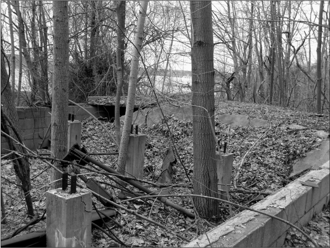
Photo 4. Northwestern end of foundation with floor joist piers and concrete slab floor, facing west.
