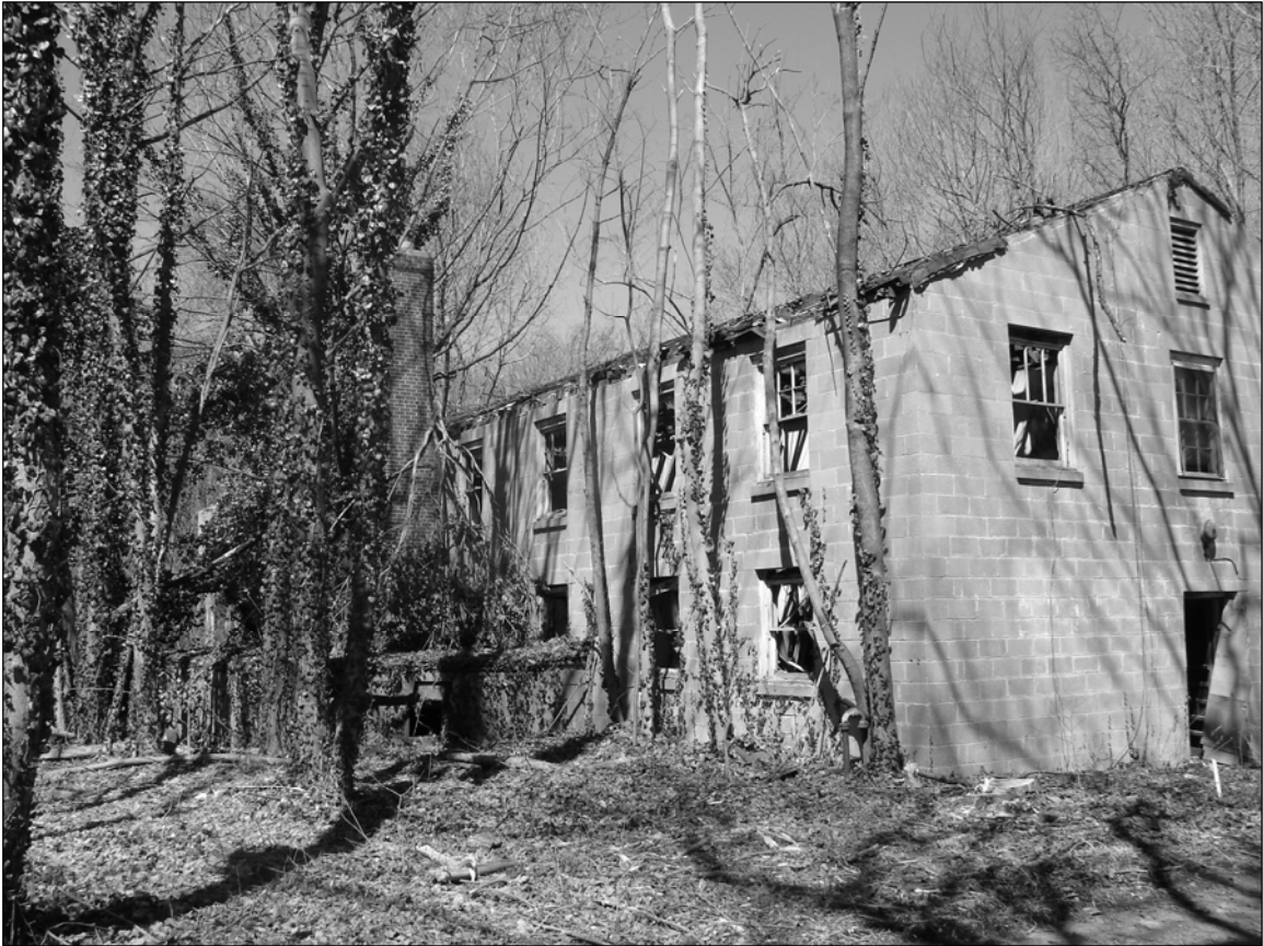
Photo 3. Southeastern end (right) and southwestern side including dependency containing boiler room (left). Facing north.
