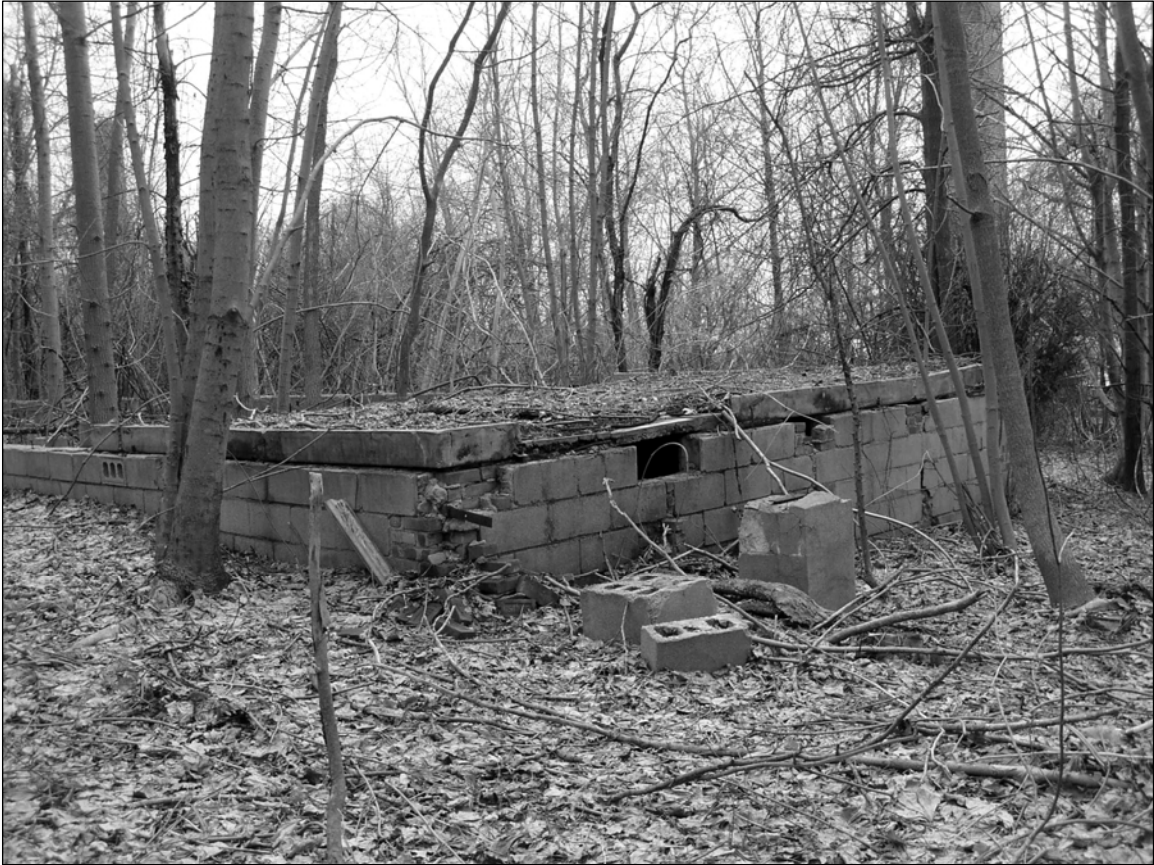
Photo 5. Concrete slab floor atop foundation wall at western end of ruin, facing southeast.
