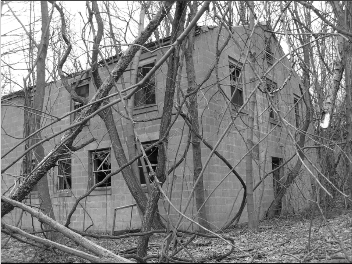
Photo 2. Southeastern end of building, showing principal façade (right) and portion of southwestern side (left). Facing north.
