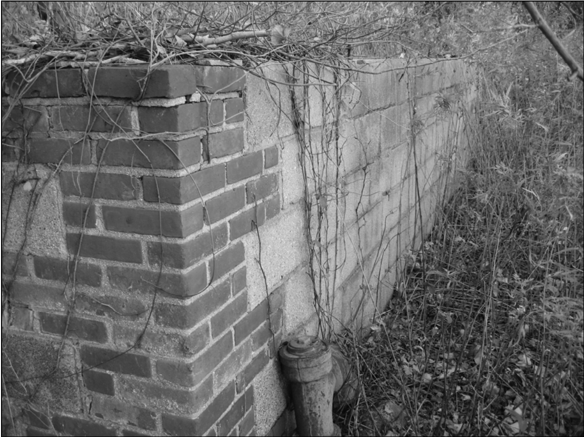
Photo 2. Building foundation, detail at southwestern corner, showing use of brick and concrete blocks. Facing southeast.
