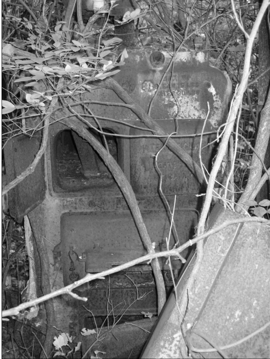
Photo 4. Mechanical system remnant in western half of foundation interior.
