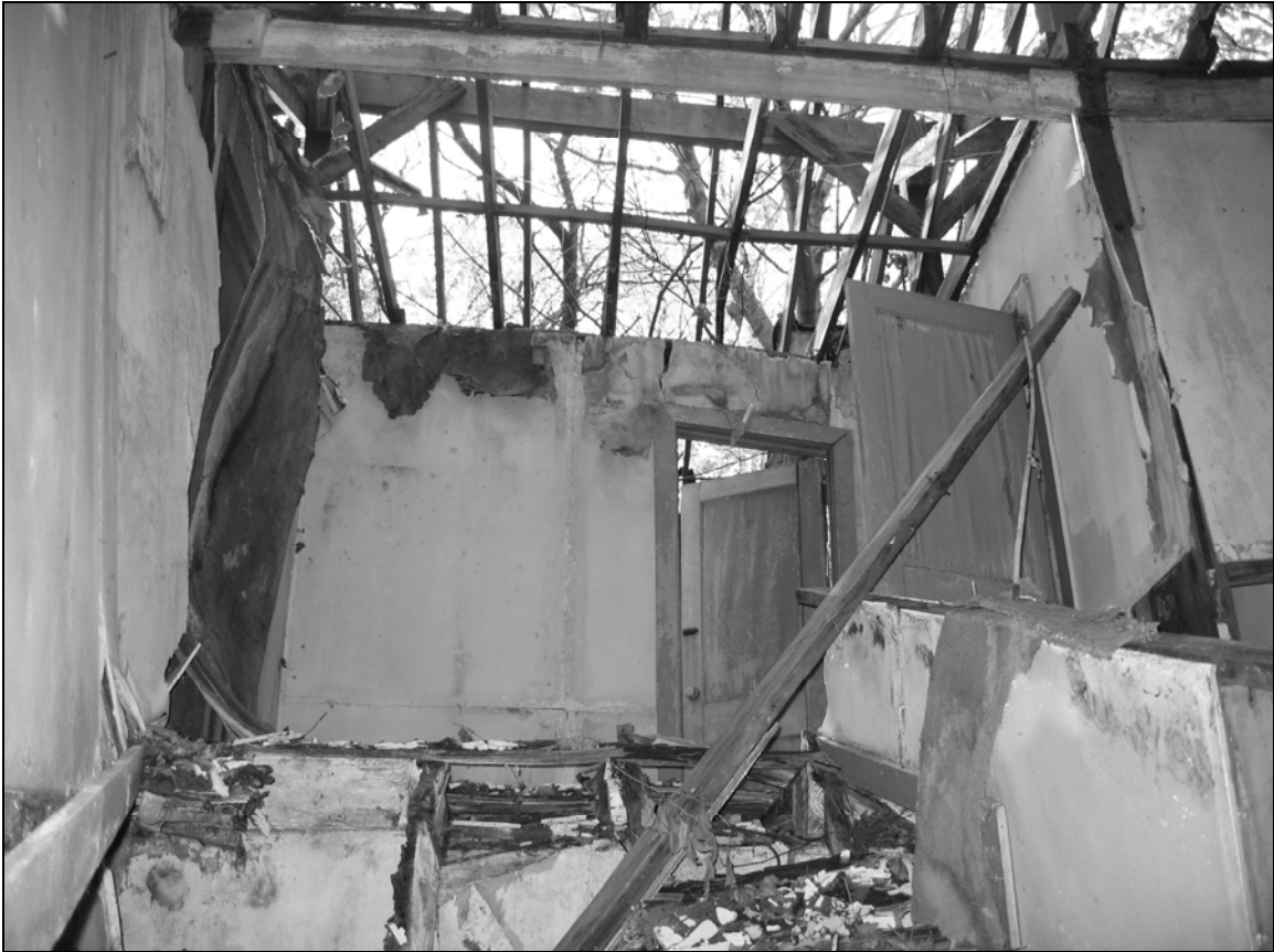
Photo 7. Partially collapsed interior, looking toward second floor corridor and exposed roof rafters.
