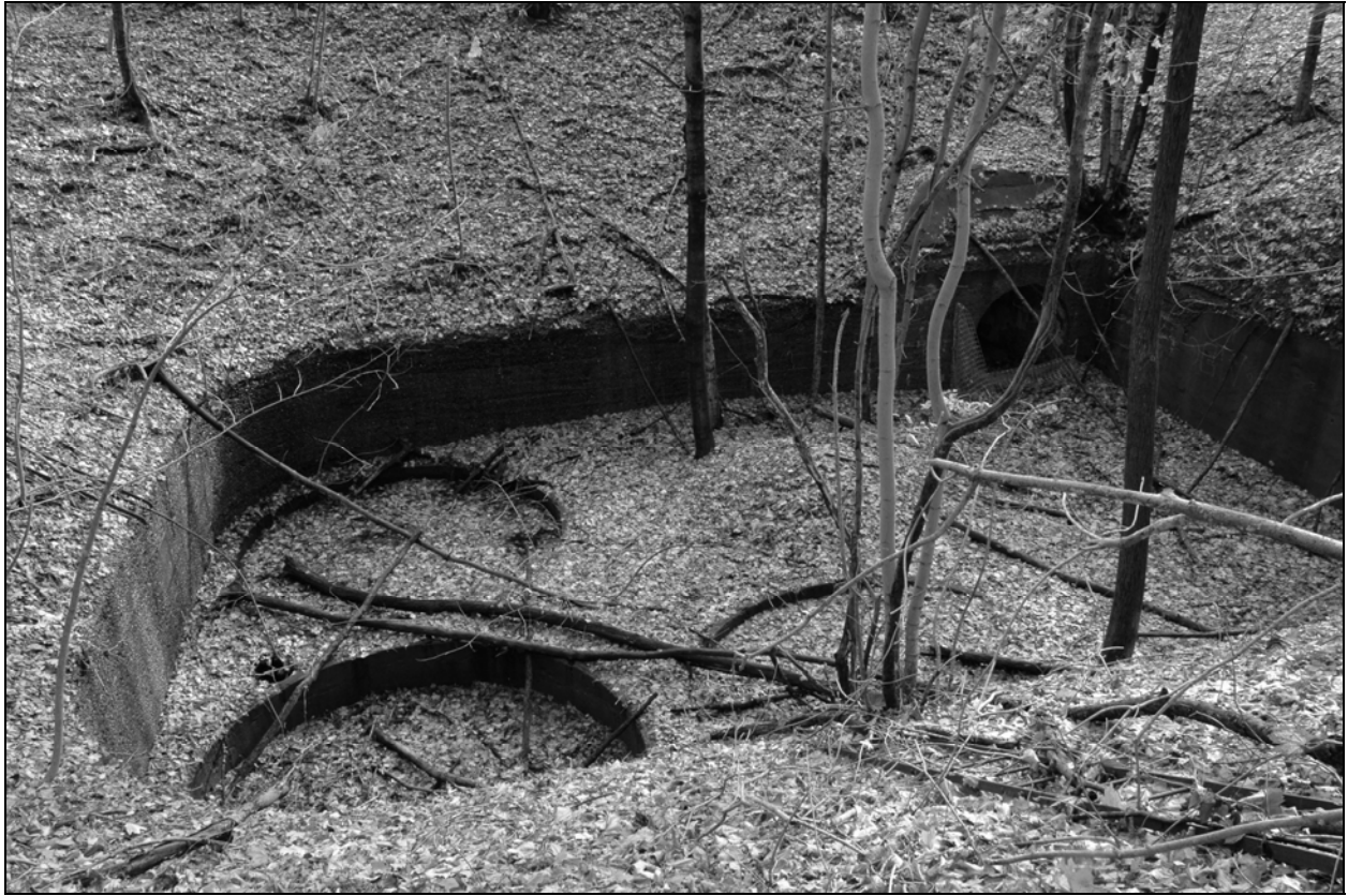
Photo 2. Battery Overton Pit B (Building 127), showing northeastern (upper left), northwestern (lower left), and southwestern (right) gun emplacements, facing southeast, covered by leaf litter and a growth of opportunistic trees.
