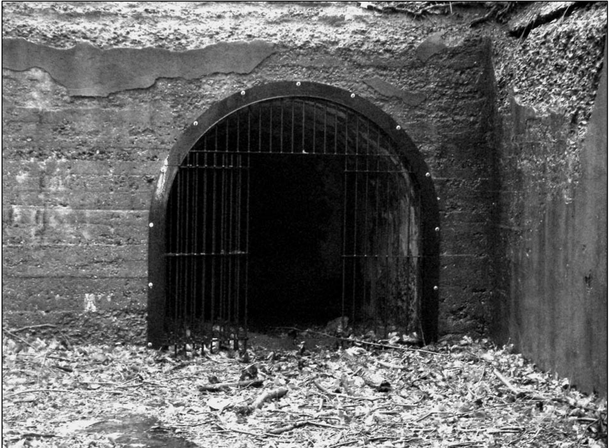
Photo 15. Gate to deter unauthorized visitors at entrance to tunnel in Battery Overton Pit B, facing southeast. Gate was installed in early 2009.
