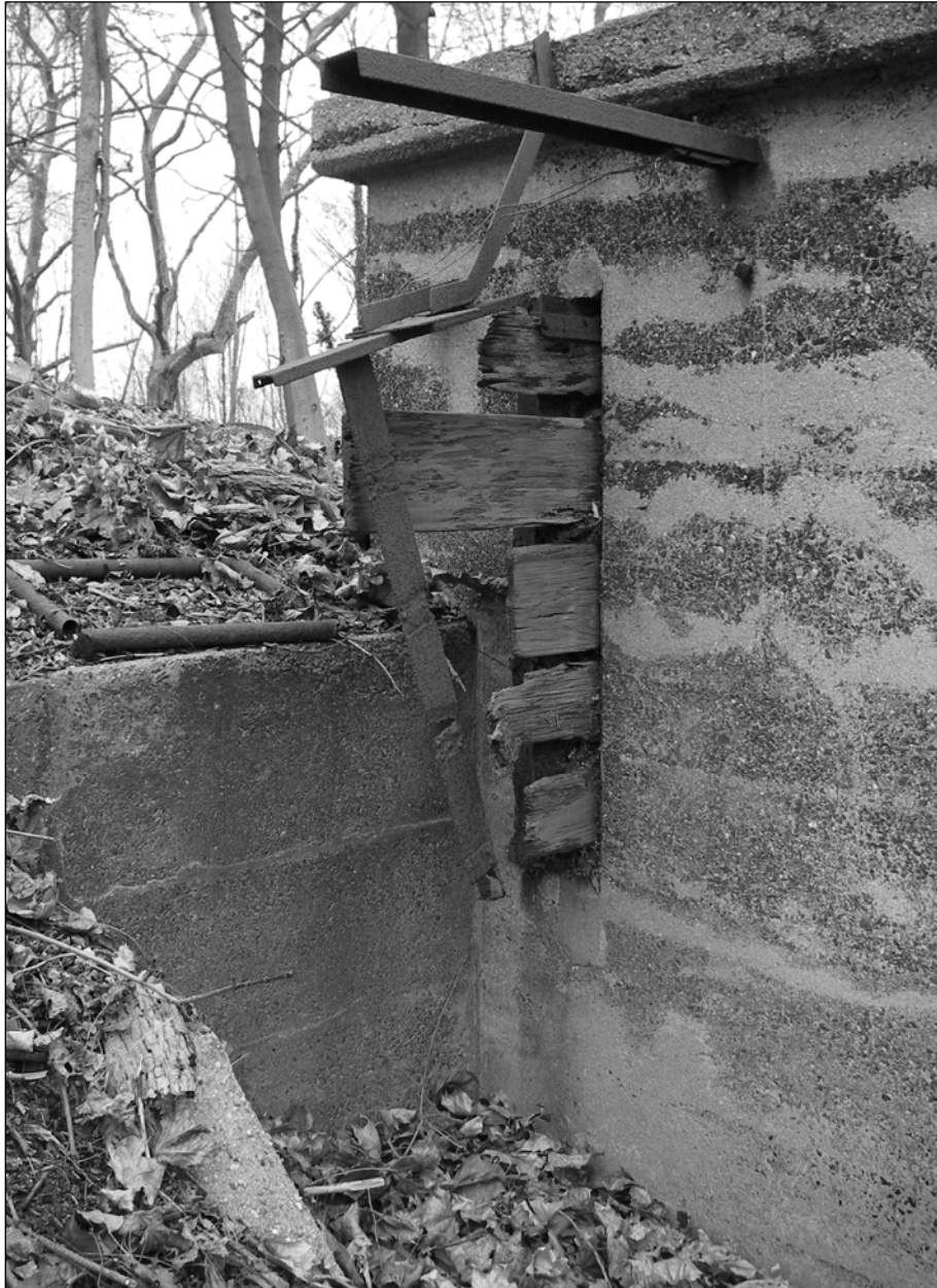
Photo 7. Eastern façade, detail: remnants of sliding blackboard and frame at southeastern corner, facing south.
