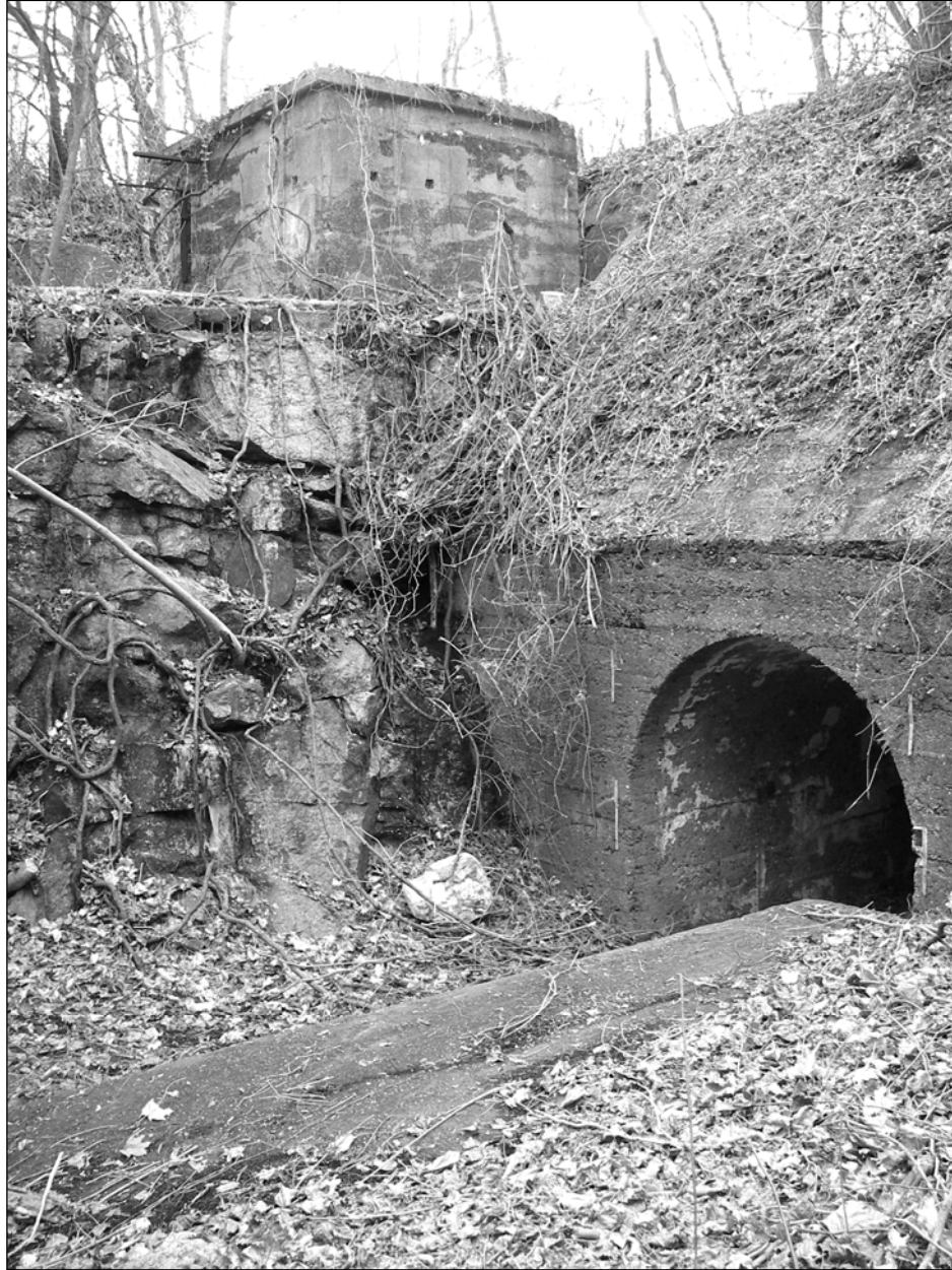
Photo 7. Southwestern corner of Battery Haskin Pit A showing unnumbered Data Booth (top left), entrance to tunnel system (right), and edge of platform for mortar emplacements (foreground), facing southwest. Note exposed bedrock of southern wall of pit (left). Photograph was taken after the opportunistic growth of trees was removed from pit floor and walls in fall 2008.
