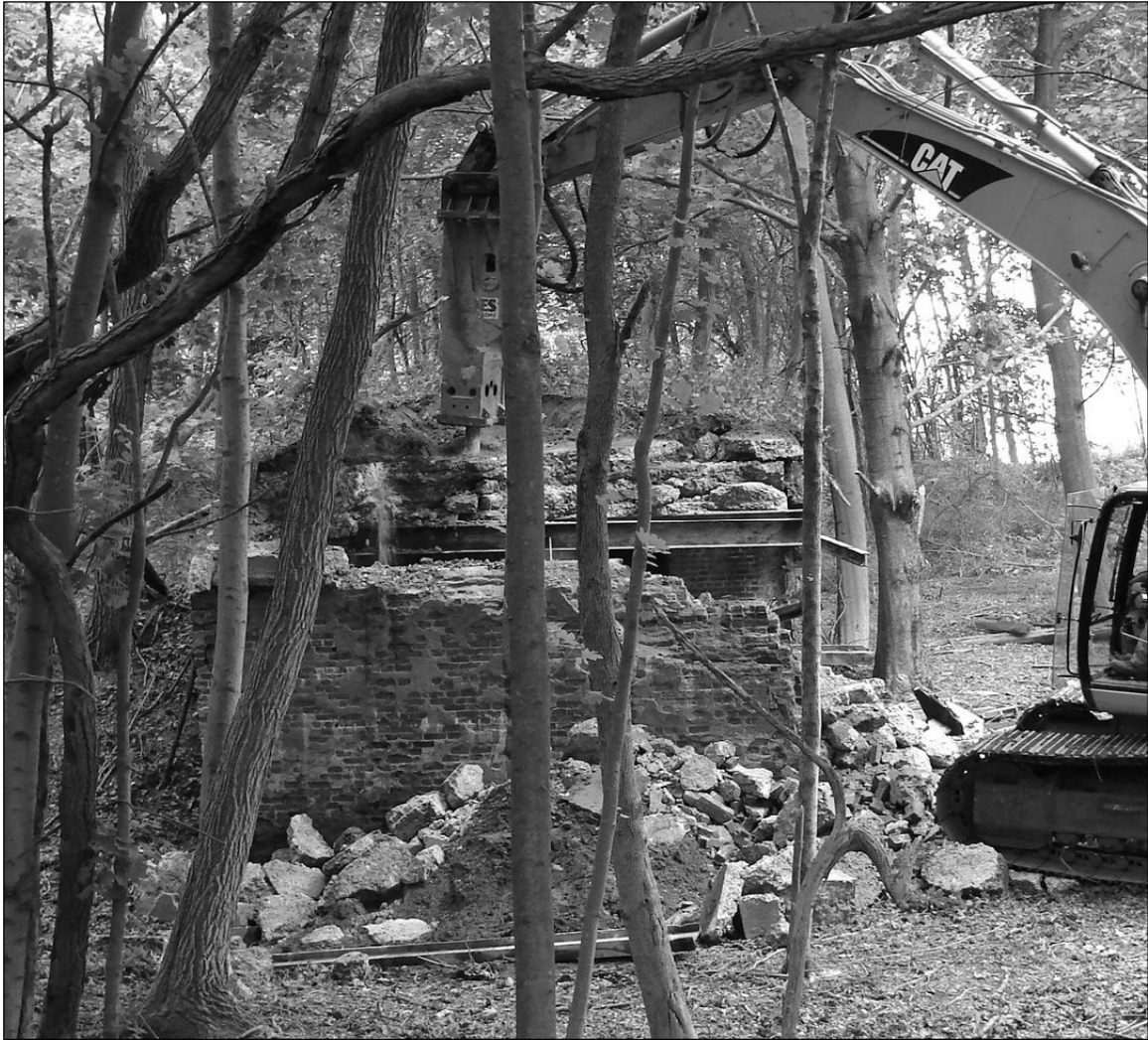
Photo 6. Demolition of Building 128 with steel beams in concrete roof exposed, facing southwest.
