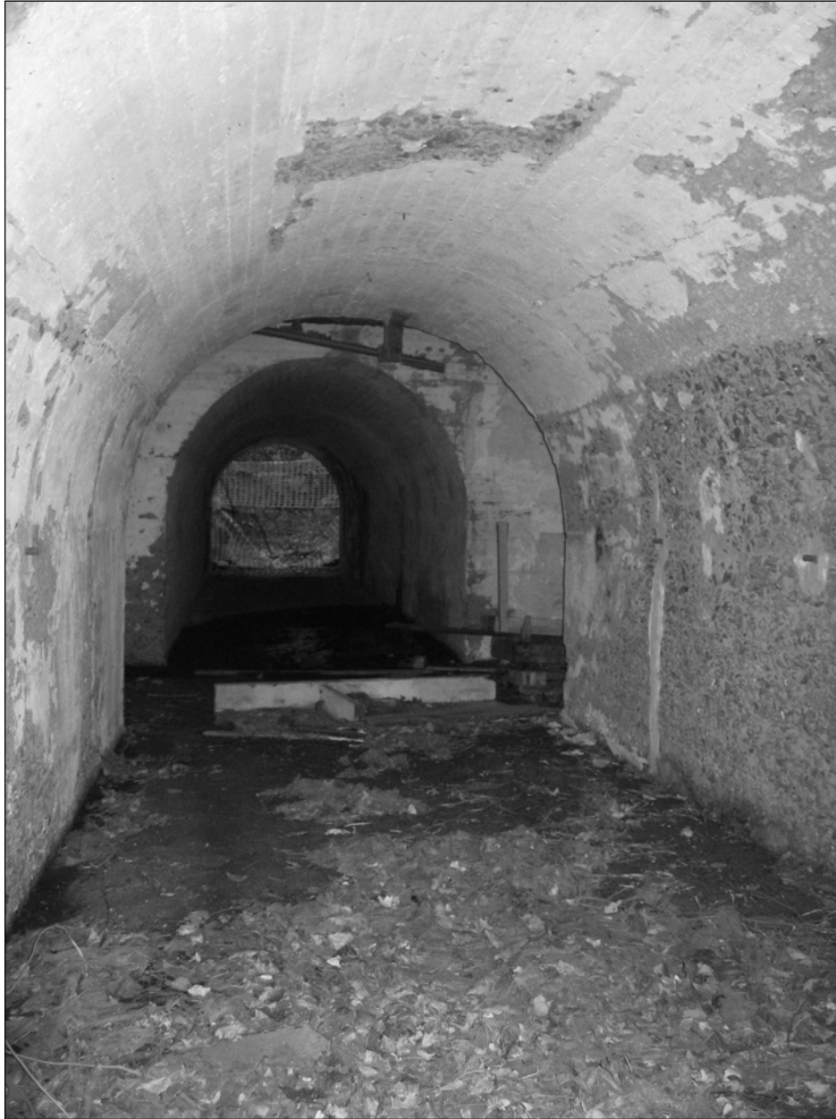
Photo 13. Haskin Lateral Tunnel, facing southeast. Battery Haskin Pit A is located at far end of tunnel.
