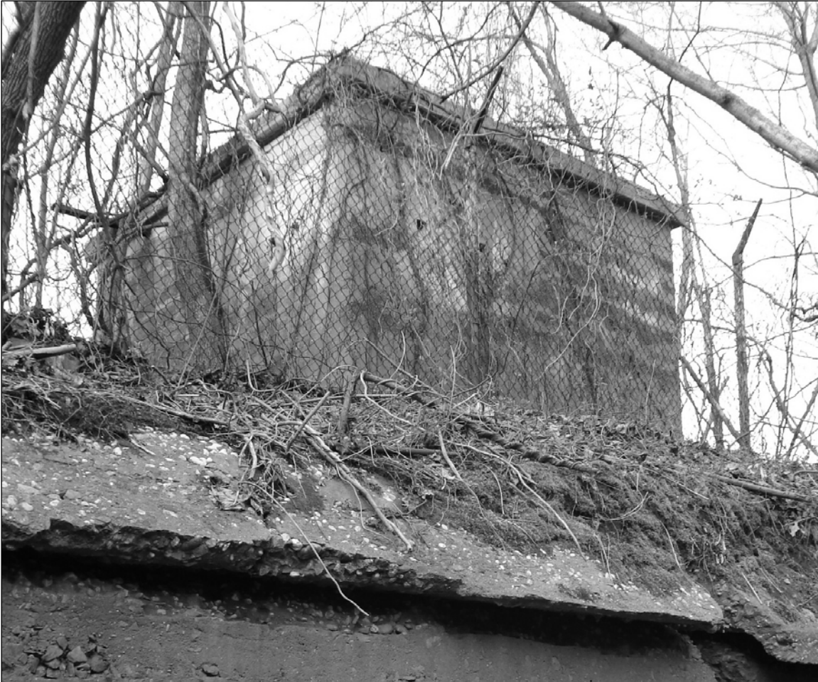
Photo 3. Northern and eastern façades as viewed from floor of mortar pit, facing southwest.
