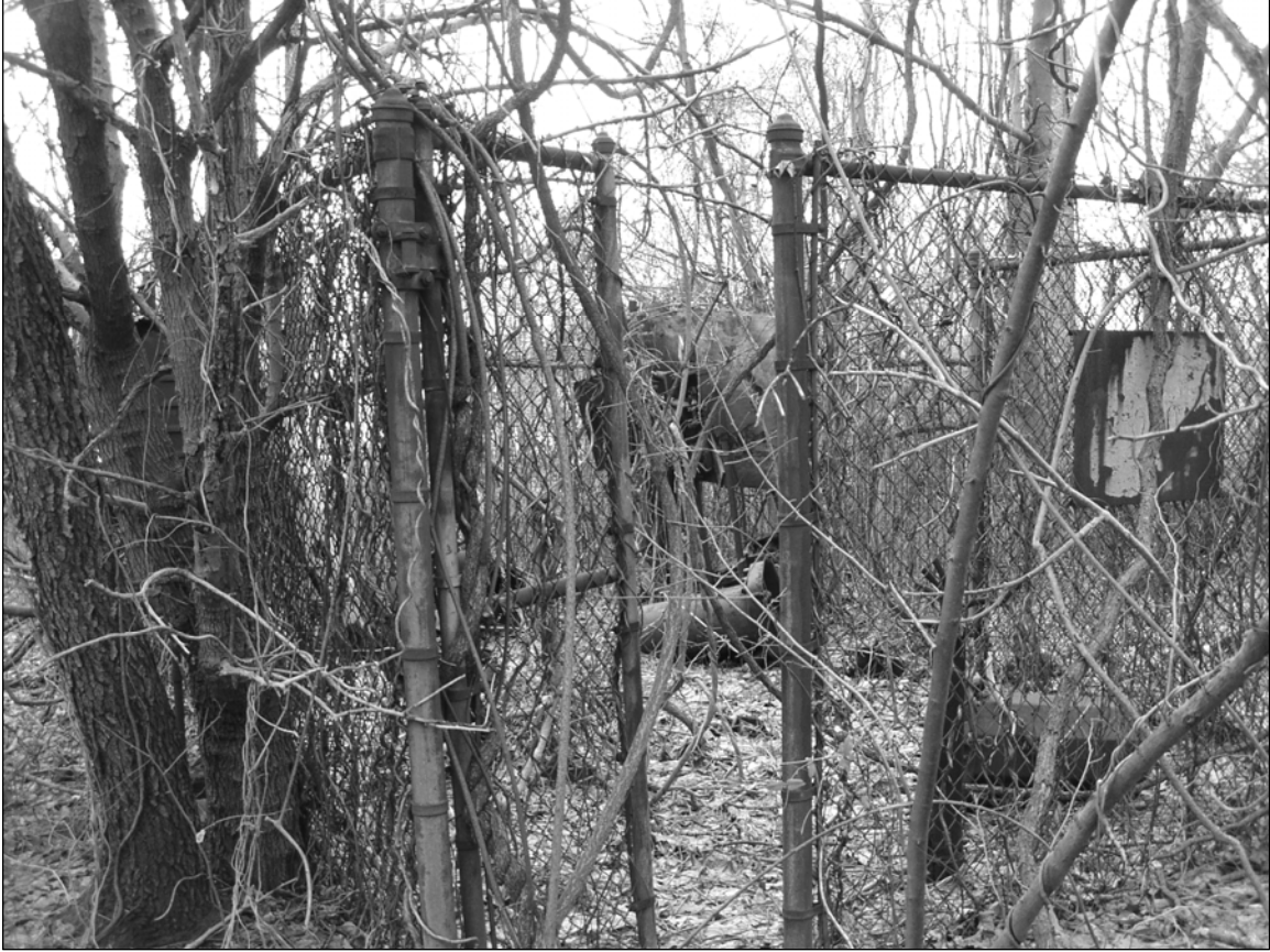
Photo 2. Gate in northeastern corner of transformer vault enclosure, facing southwest.
