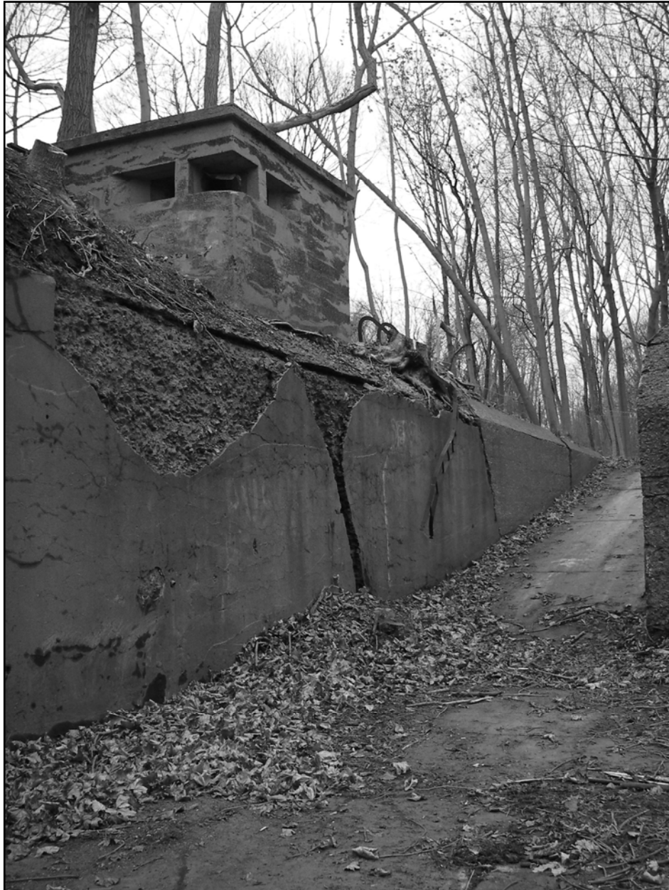
Photo 3. Building 128A and Battery Overton entrance ramp from floor of mortar pit, facing south.
