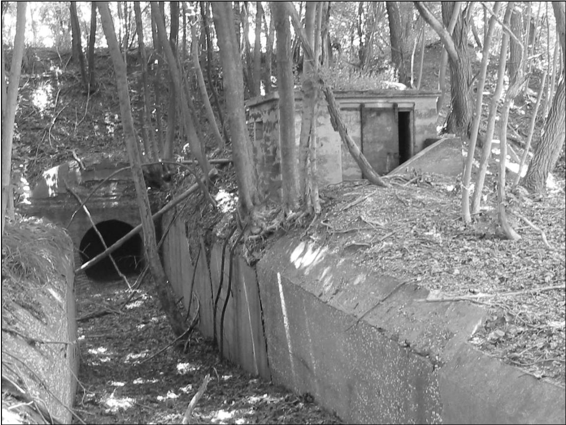
Photo 2. Building 128A (right), adjoining entrance ramp to Battery Overton (left), facing southeast. Entrance at left leads to tunnel system in the central part of the Mortar Battery.
