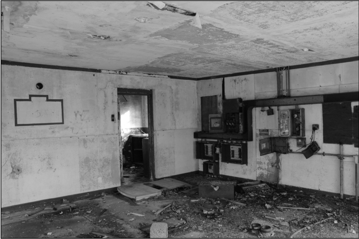
Photo 5. Main room interior, facing north. Fuse boxes and other electrical controls on northeastern wall.
