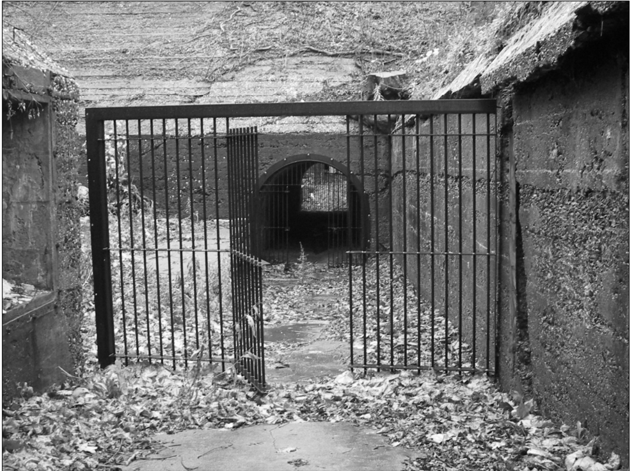
Photo 14. 14. Gate to deter unauthorized visitors at entrance to Battery Haskin Pit B, facing southeast. Gate was installed in early 2009.
