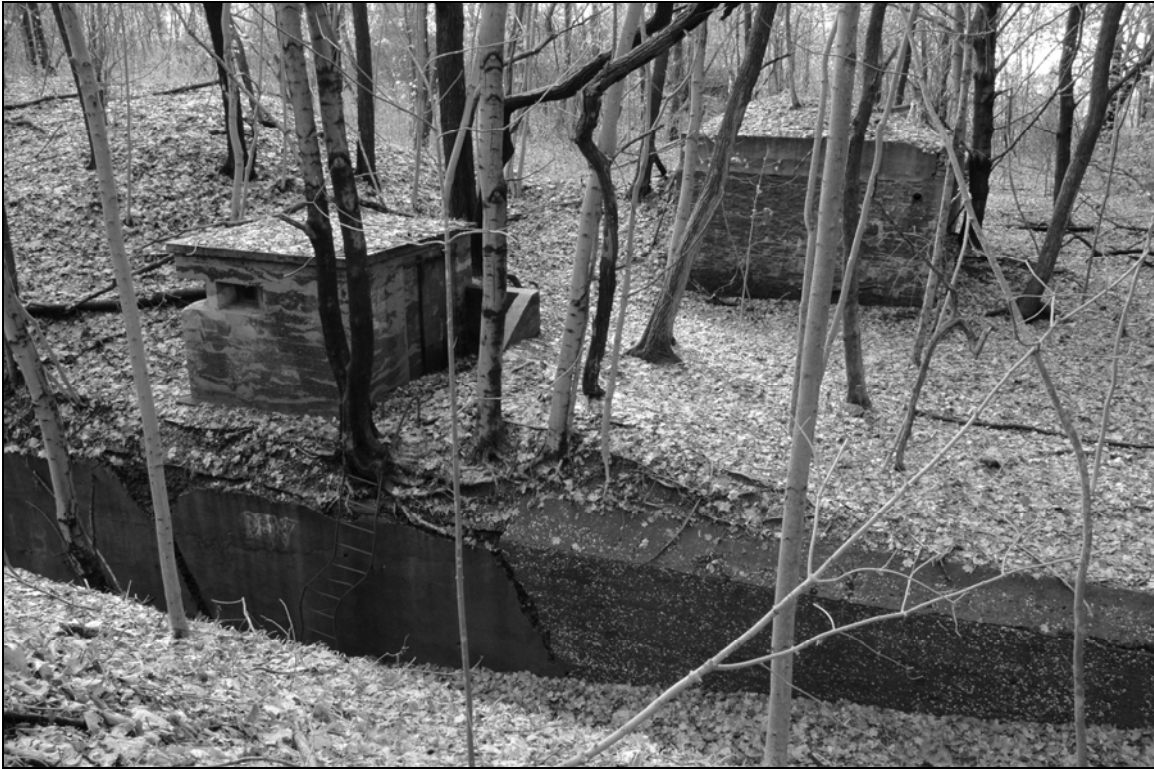
Photo 1. Setting of Building 128 (right), facing southwest. Building 128A is at left and the entrance to Battery Overton Pit B is in the foreground.
