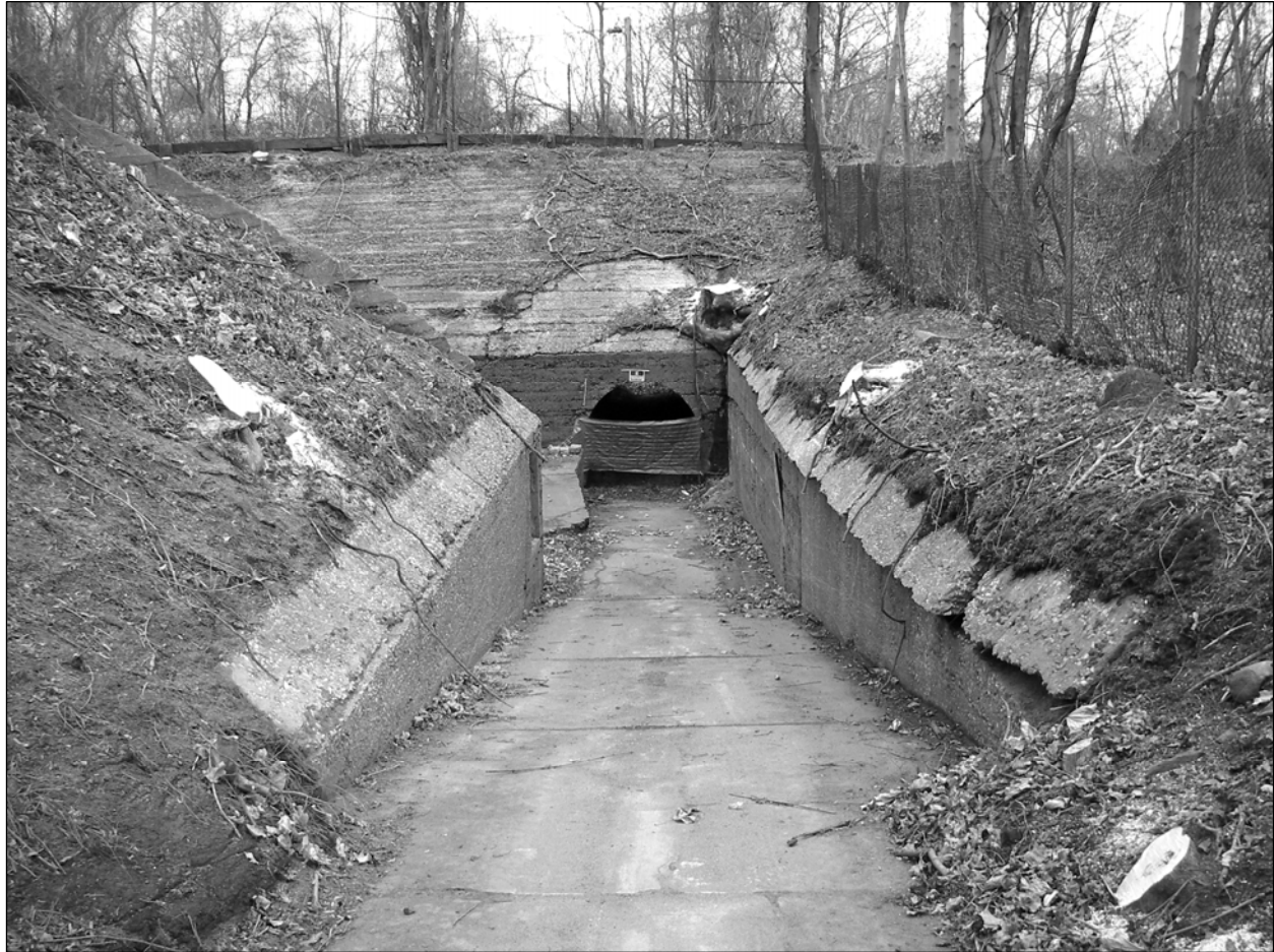
Photo 5. Entrance ramp to Battery Haskin Pit B after removal of opportunistic growth of trees in fall 2008, facing southeast. The Mortar Battery Data Booth associated with this pit (Building 127B), which formerly stood to the right of the pit's near corner, had been demolished by the time of this photograph.
