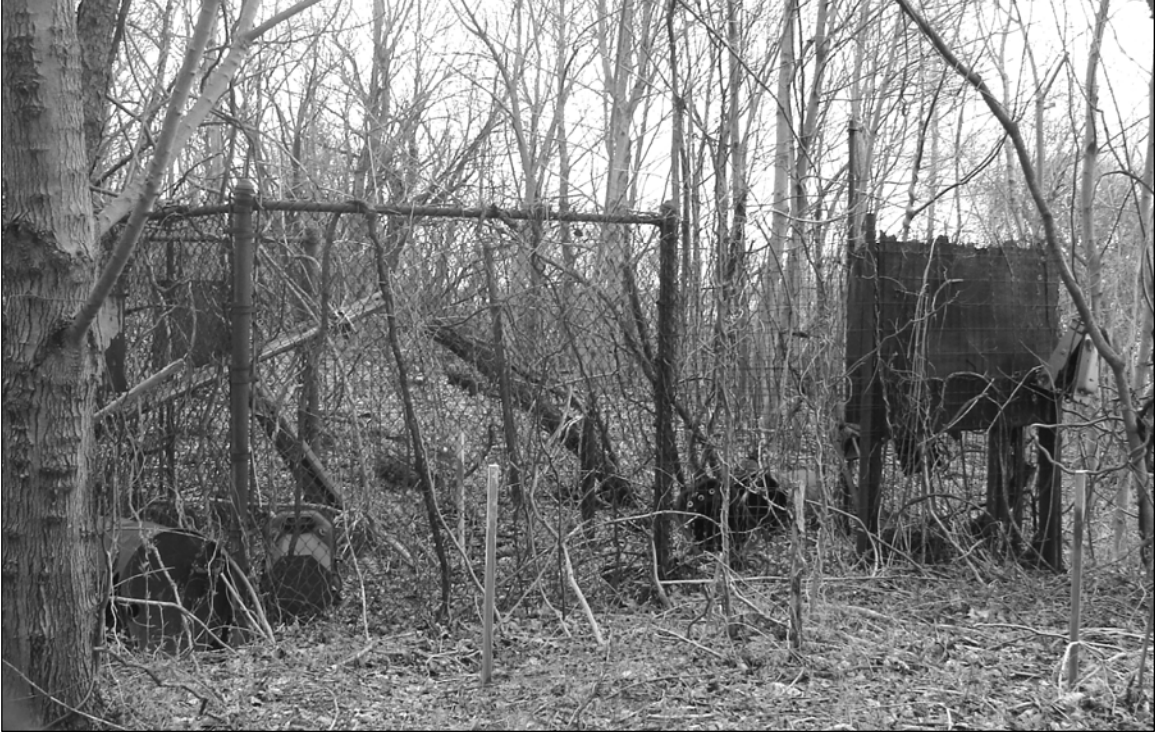
Photo 3. Northwestern side of transformer vault enclosure, facing south.
