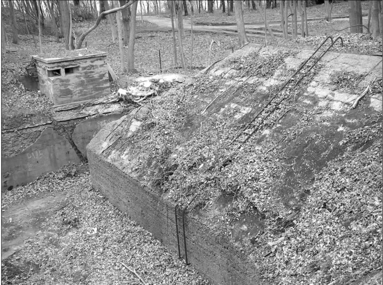
Photo 4. Western wall of Battery Overton Pit B (right) with Mortar Battery Data Booth (Building 128A) (left), facing southwest after removal of opportunistic growth of trees on pit walls and floor in fall 2008. Note steel ladder attached to pit wall (center right). Mortar Battery Powerhouse (Building 128), which formerly stood about 30 feet behind the data booth had been demolished by the time of this photograph.
