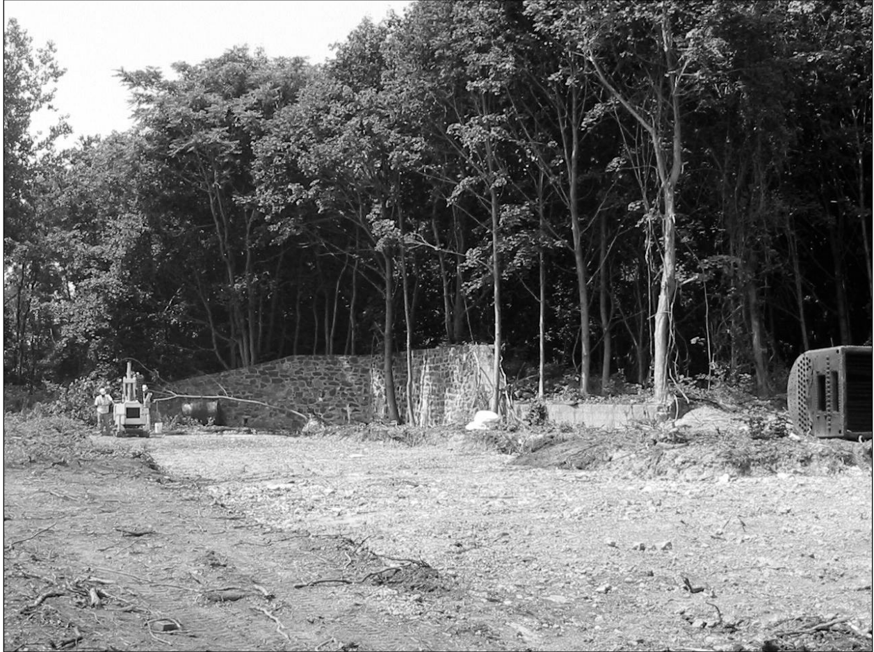
Figure 9. View across footprint of south wing of Ordnance Storehouse/Laundry (Building 110) after its demolition, facing southwest. Photograph looks toward Pistol Range, located in the woods, which occupies the former location of Battery Overton Pit A (demolished 1941-1942). Stone wall at center-left was constructed in ca. 1939 as a retaining wall when the south wing of Building 110 was built into the then-extant northeastern corner of the mortar pit earthwork.
