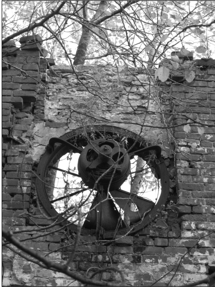
Photo 9. North wing, detail of ventilation fan in eastern gable peak. View from interior facing east.
