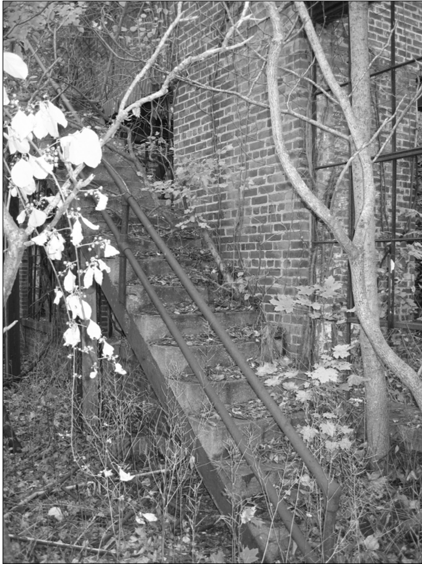
Photo 12. Eastern side of east wing, detail of concrete and steel stairway to second-story apartment, facing southwest.
