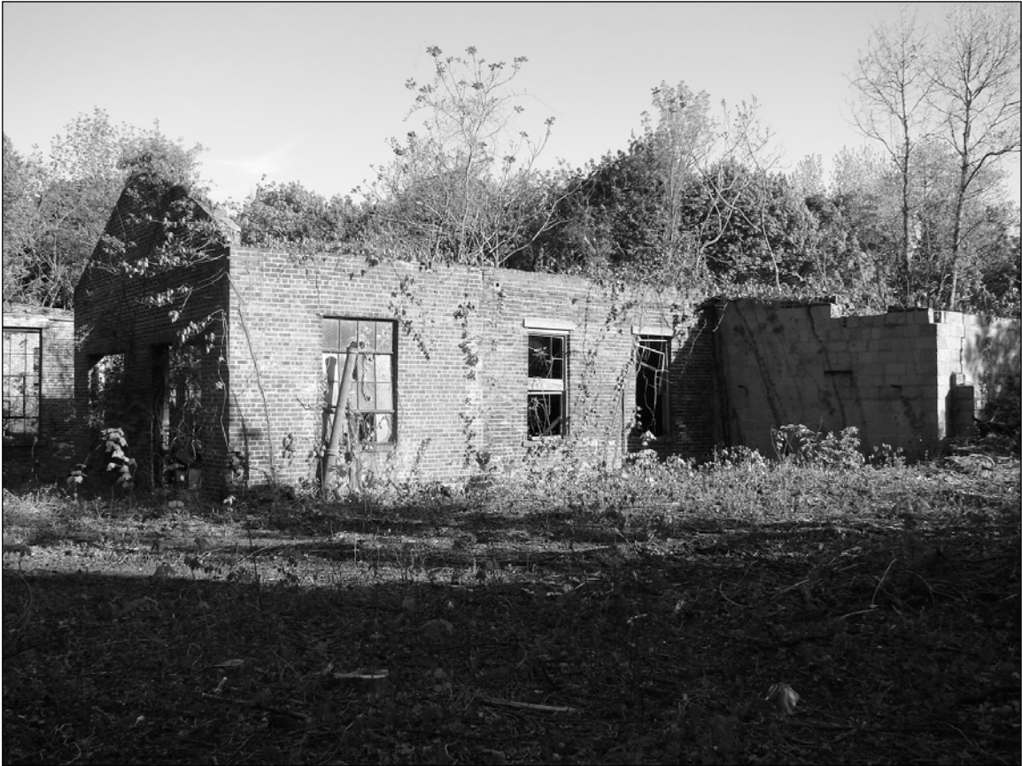
Photo 6. Southern and eastern façades, including concrete block coal bunker ell, shortly before demolition, looking west-northwest.
