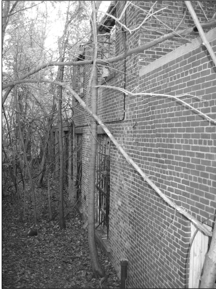
Photo 15. East wing, western façade, facing south from vicinity of southwestern corner of one-story addition.
