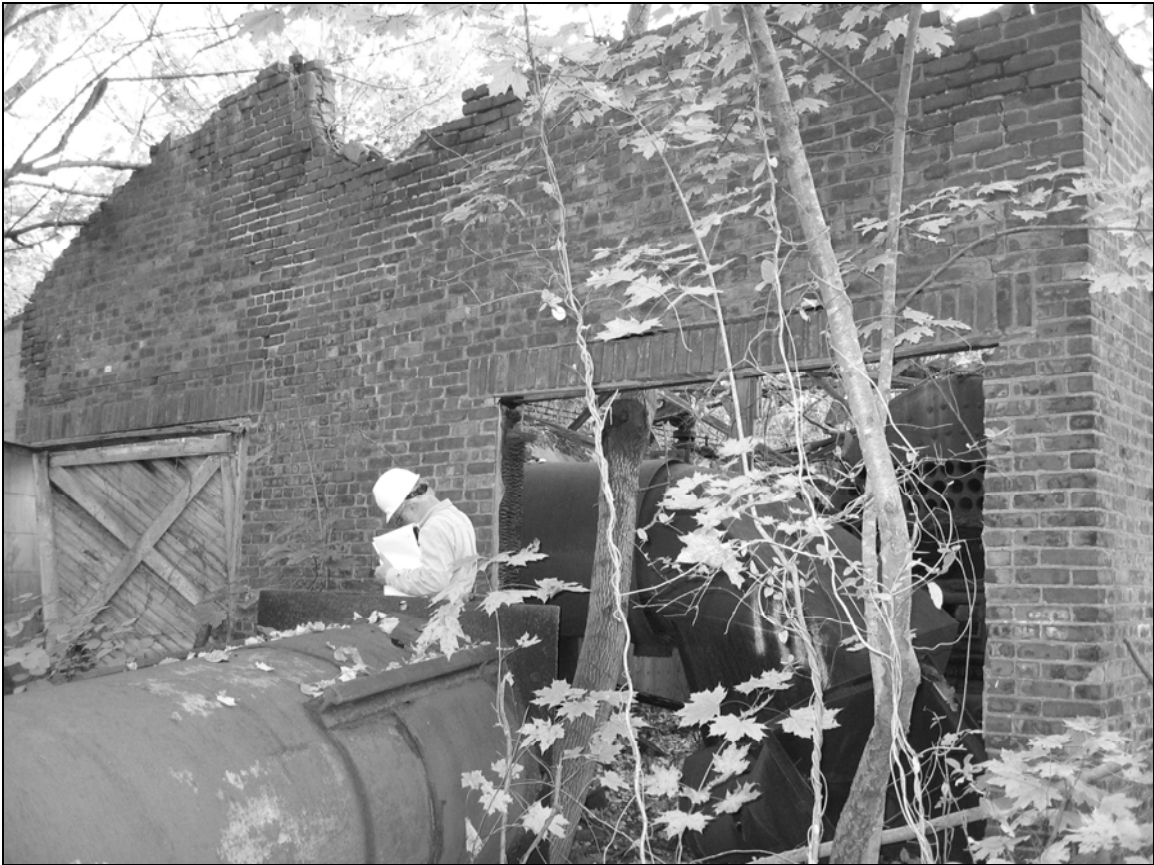
Photo 2. Main section of northern façade, facing south. Collapsed smokestack in foreground.
