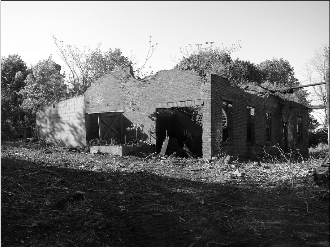
Photo 4. General view of Building 114 shortly before demolition, showing northern and western façades.
