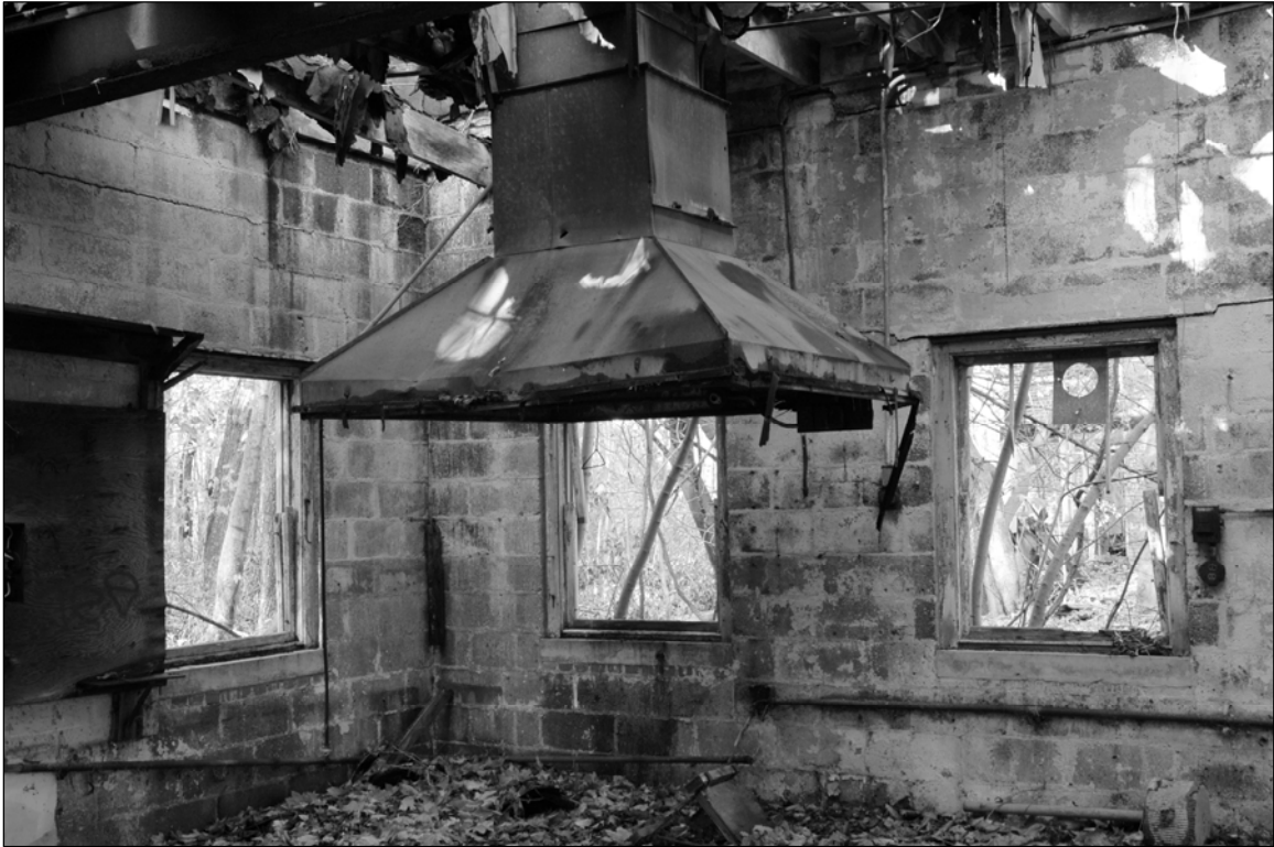
Photo 2. North wing, one-story addition at west end, interior with fume hood, facing northwest.
