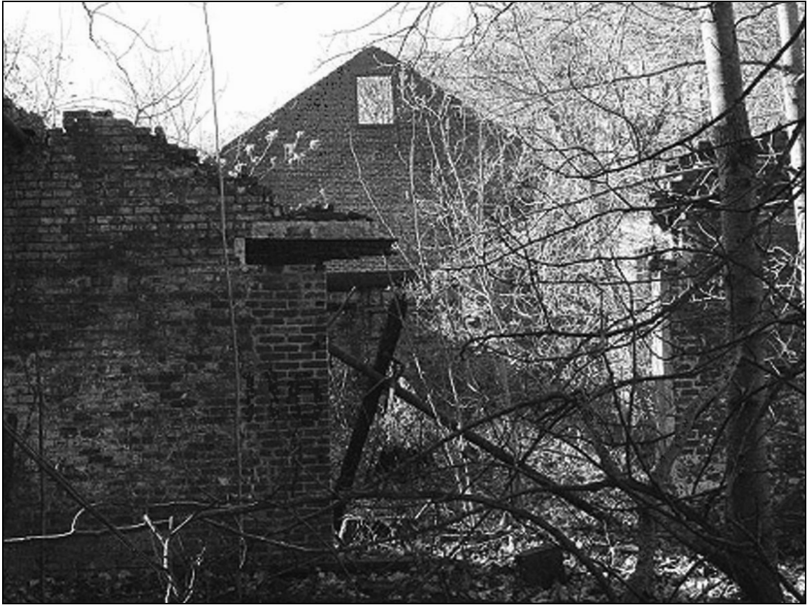
Photo 1. Interior, east end of north wing, facing south into east wing. Gable of two-story addition is visible at top center.
