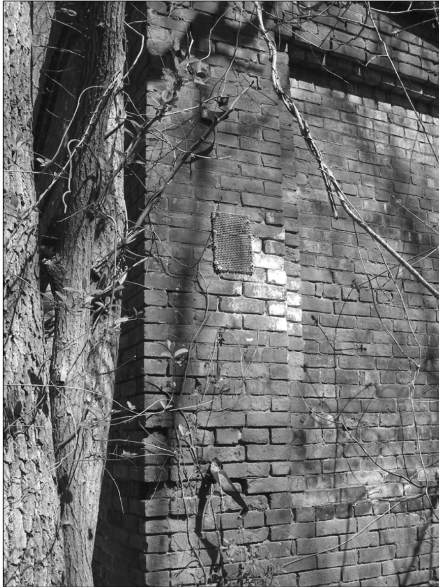
Photo 4. Exterior, northwestern corner, detail including coarse bronze screen covering opening in wall, facing east-southeast.
