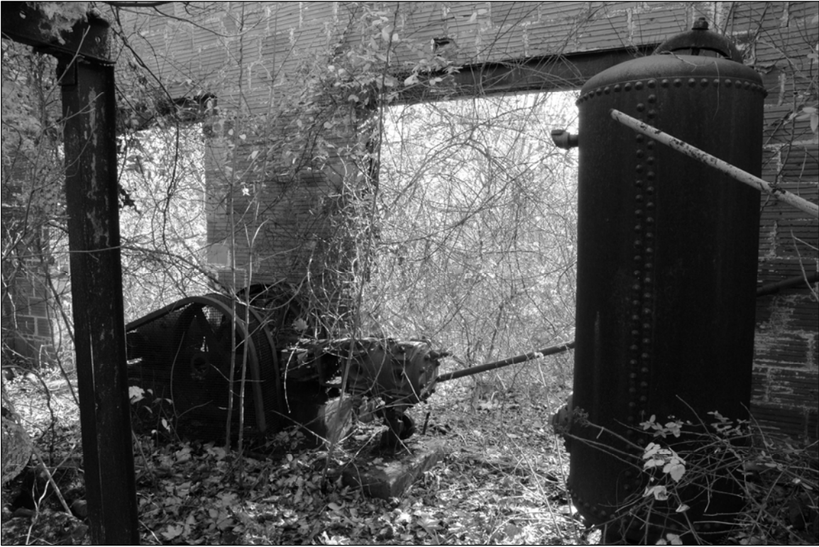
Photo 10. Southern section of building, interior, showing ruins of boiler system and other machinery.
