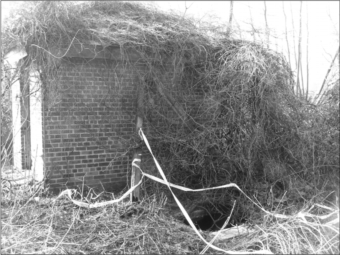
Photo 2. Northern façade, facing south, with open panel above underground vault visible at lower right.
