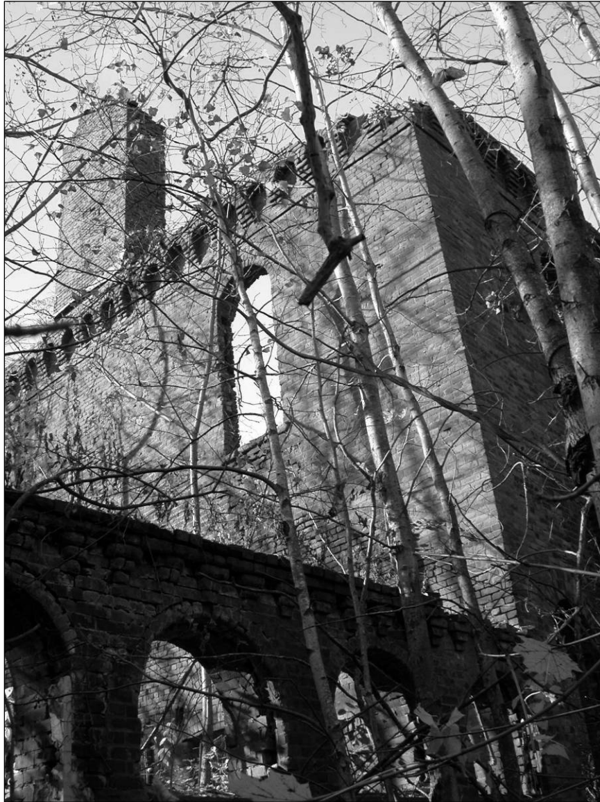
Photo 14. Eastern façade of center tower, showing chimney and cornice, with lavatory block below, facing southwest.
