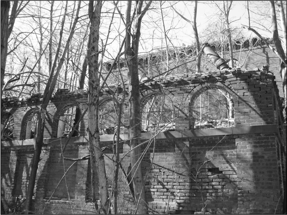
Photo 13. Eastern façade of lavatory block with cornice of center tower in background, facing west.
