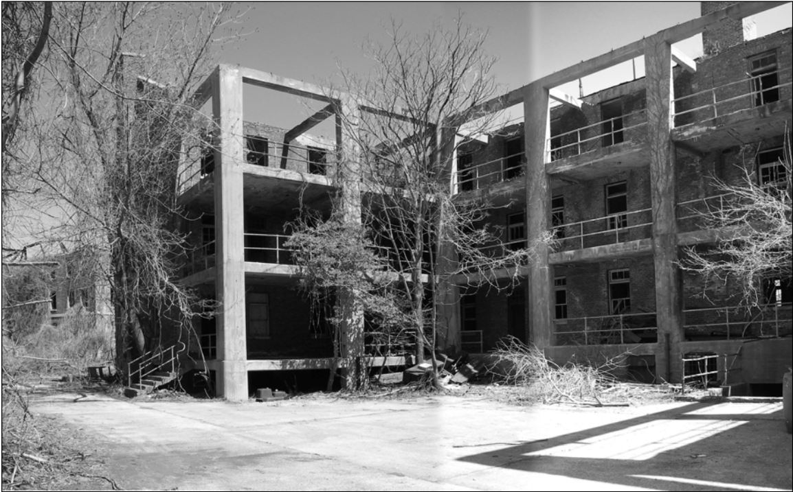
Photo 8. Mosaic photograph of courtyard on western side of building, showing porches, looking northeast.
