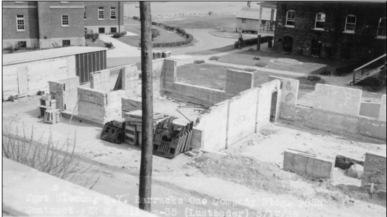
Figure 6. Foundation work for rebuilding of Building 61 after 1937 fire. Photo taken May 17, 1939. View southeast. Building 60 is at upper left. Record Group 77, National Archives, College Park, MD.
