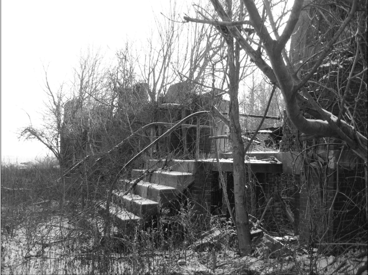
Photo 7. Concrete stairway leading from center of hall, northern side of building, fifth bay from eastern end, facing west.
