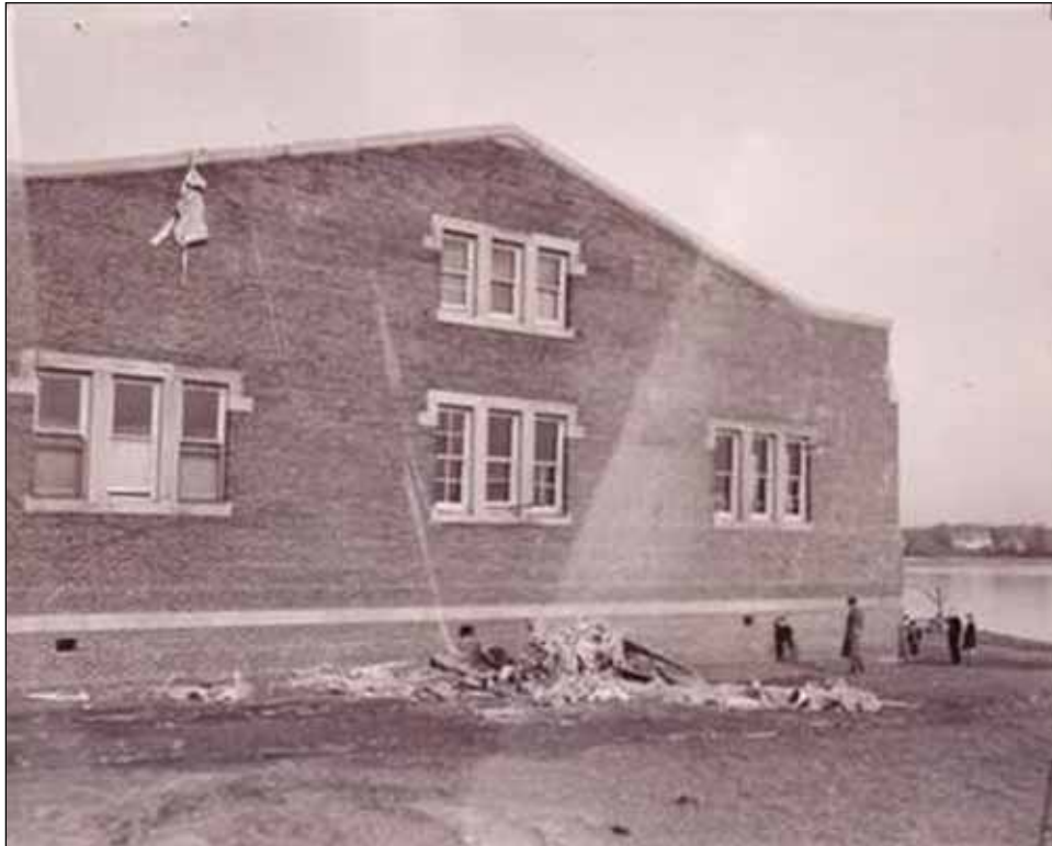
Figure 3. Rear façade (east end) of Building 57 following crash of light airplane, March 1936. View west-northwest. Fort Slocum Alumni and Friends Collection, Michael A. Cavanaugh, Los Angeles, CA, custodian.
