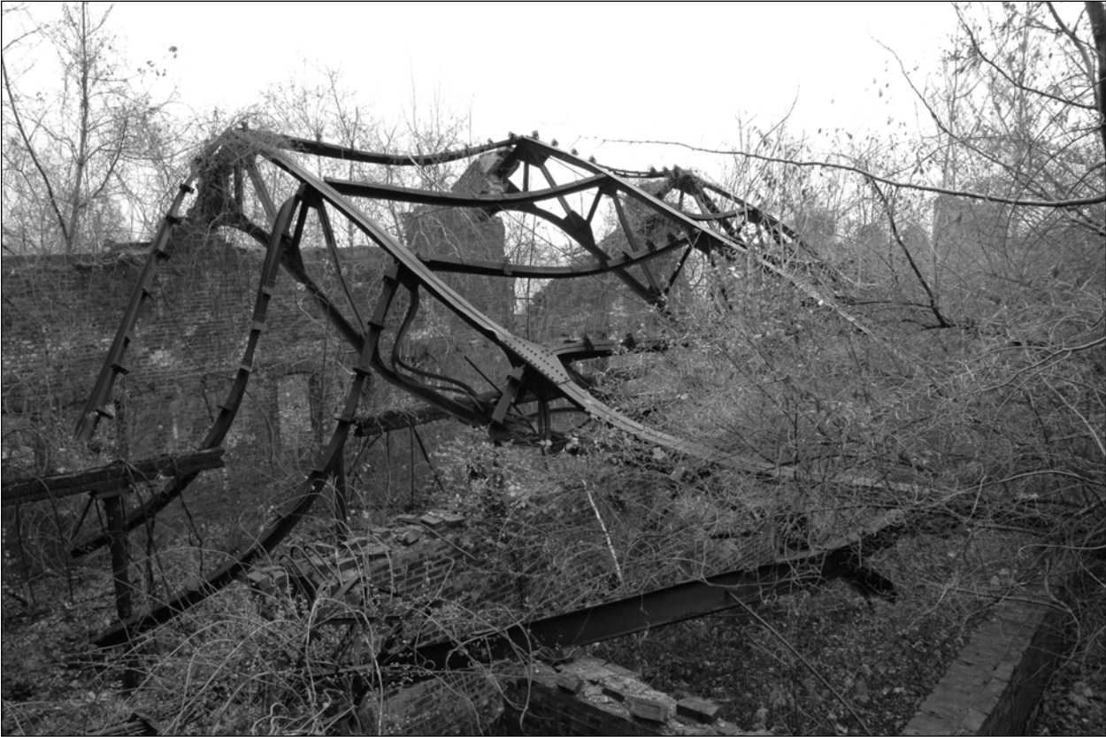
Photo 9. Hall interior, detail showing collapsed roof trusses.
