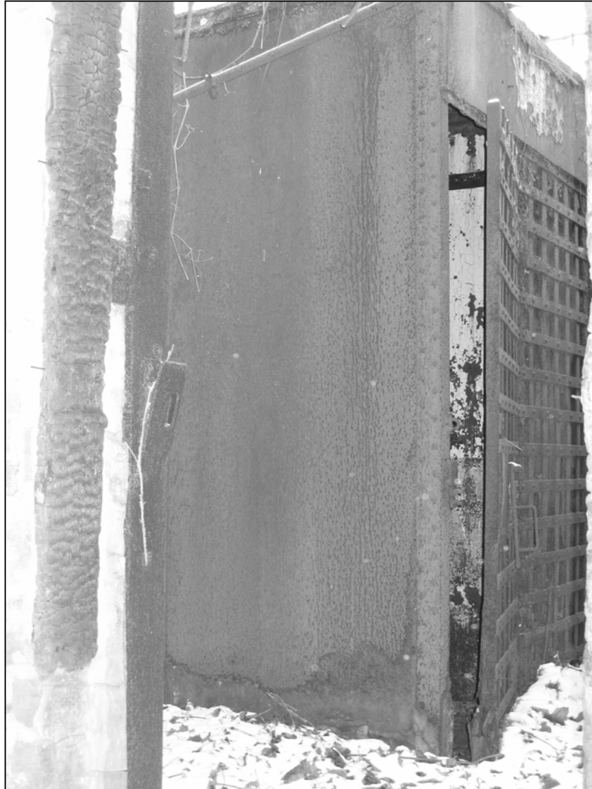
Photo 5. Ruin of steel cell in building interior.
