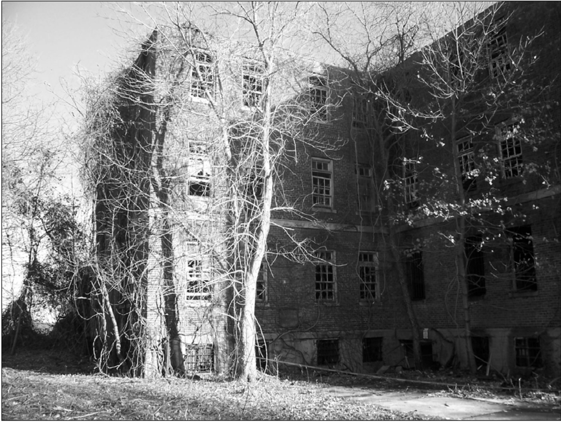
Photo 5. Western façade at northern end of building (left) and northern façade of north wing, facing southeast.
