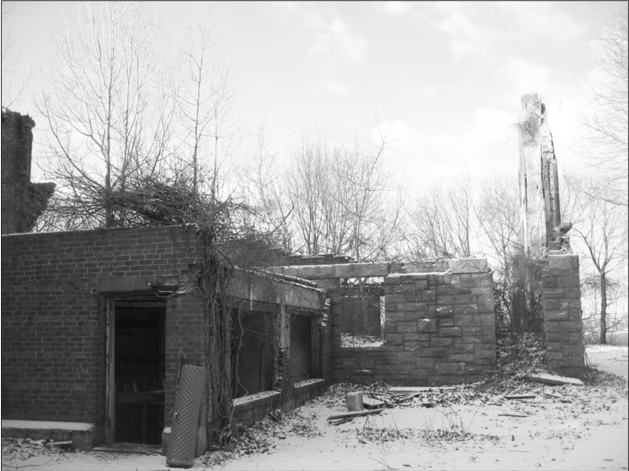
Photo 14. Northern ends of boiler room-utility area and rear north wing, facing west.
