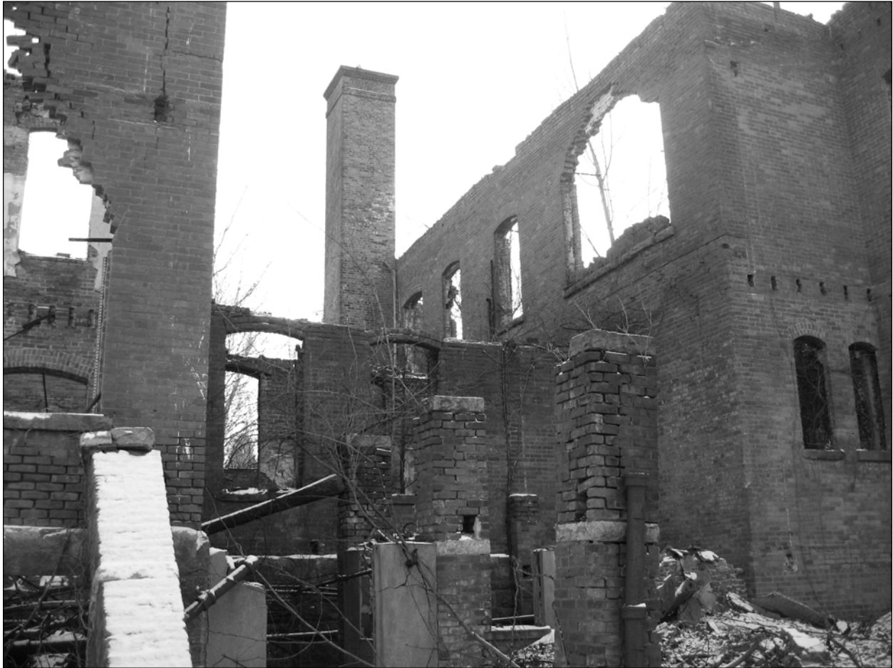
Photo 18. Southwestern corner of rear north wing (left), northern side of front west wing (right), and connecting corridors and porch piers (center), facing southeast.
