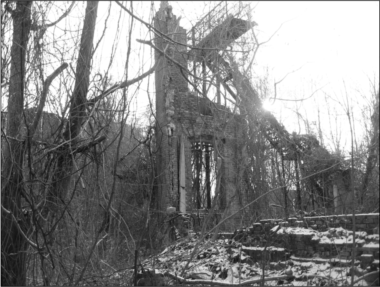
Photo 9. Northeastern corner of front east wing with adjoining self-supporting steel fire escape, facing southeast.
