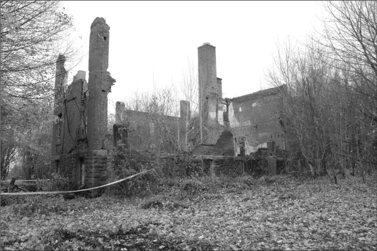
Photo 16. Ruins of rear north wing, facing southeast.
