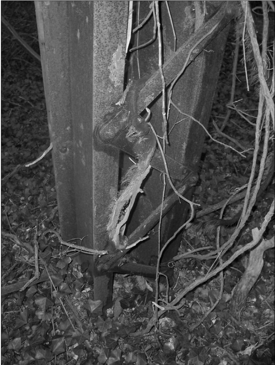
Photo 5. Detail of base of tower, showing the parallel pieces of channel iron comprising the leg, which are joined by riveted zig-zag braces.
