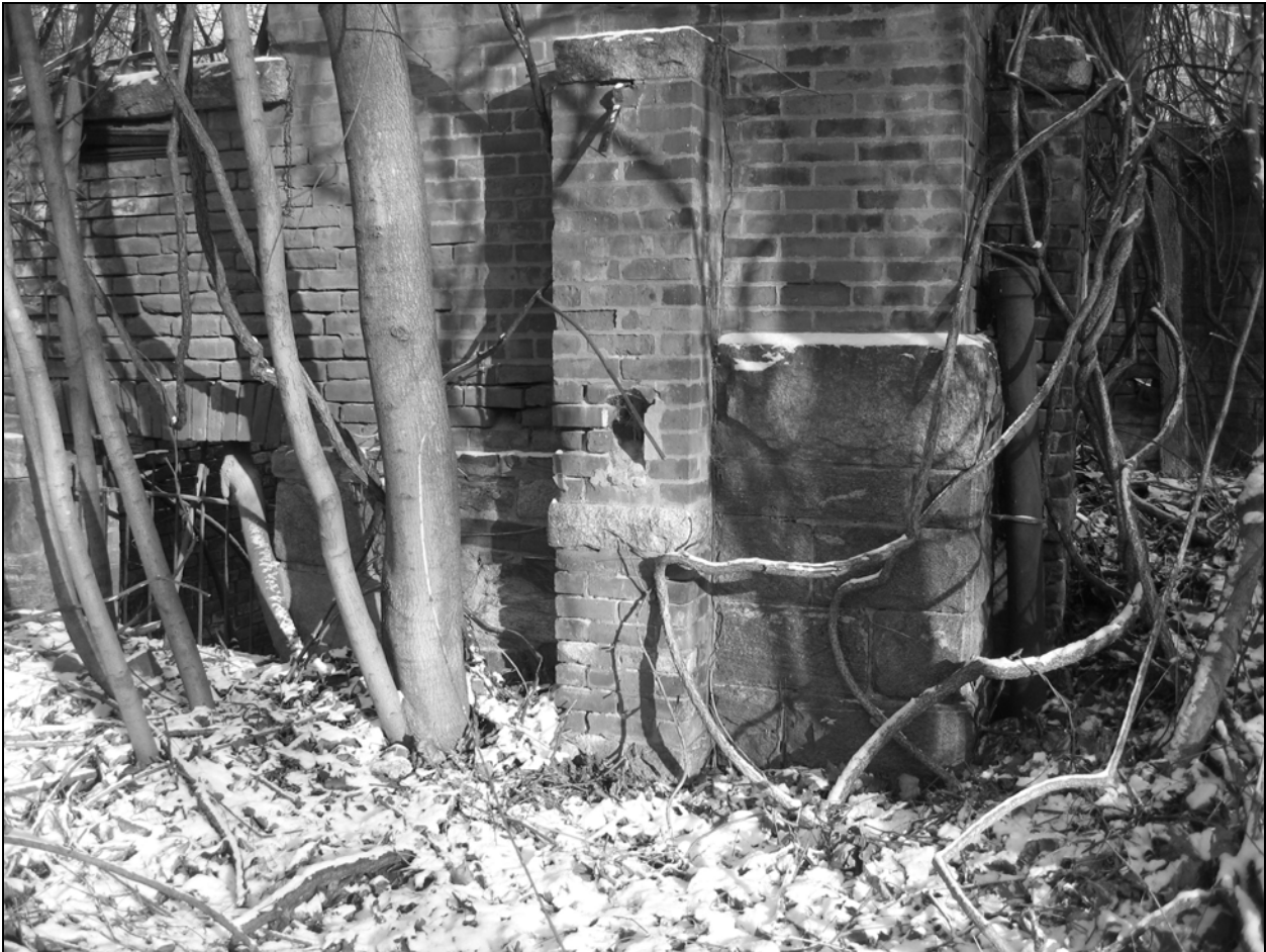
Photo 7. South façade, detail of southeastern corner of front east wing, facing north.
