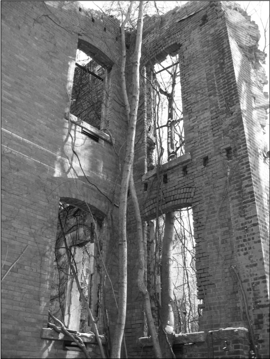
Photo 4. South façade, detail: east end of front west wing at west wall of central pavilion, facing northeast.
