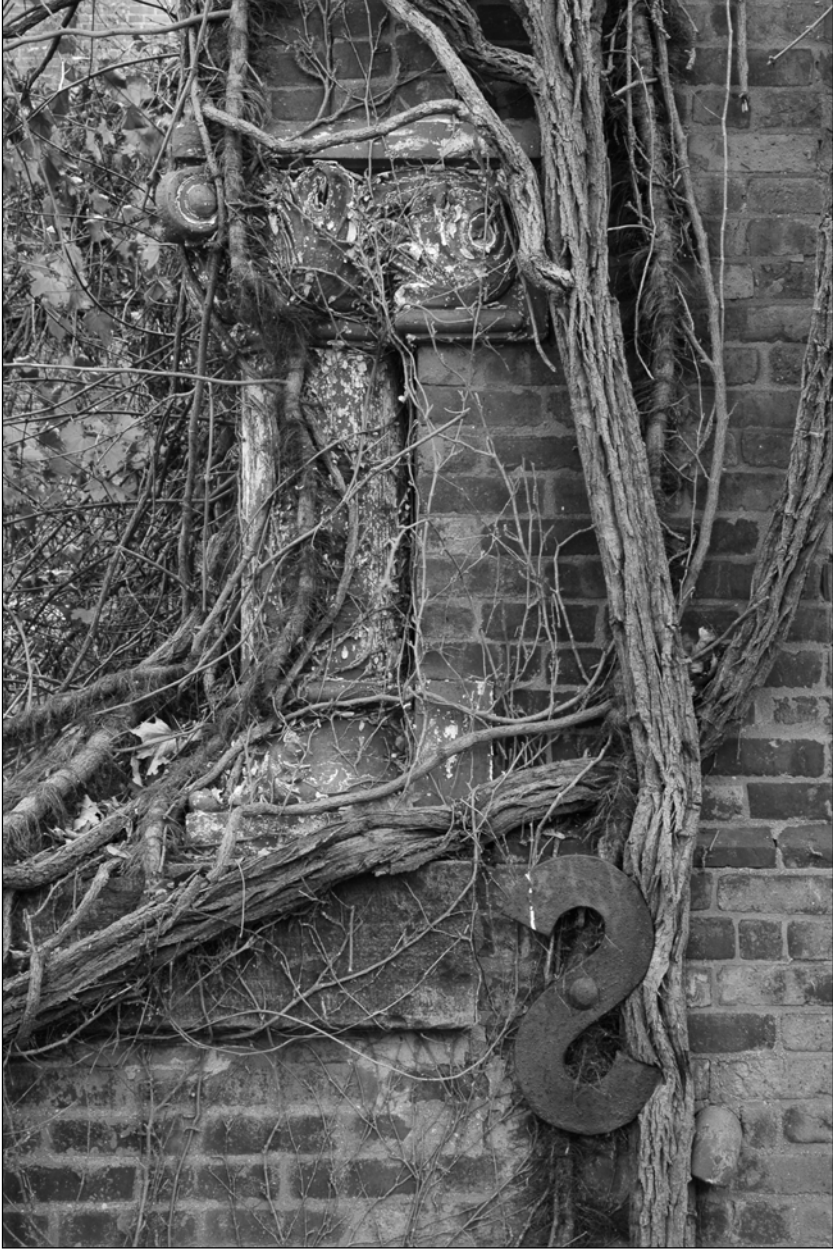
Photo 3. Northwestern façade of tower, detail, showing engaged terra cotta dwarf column and S-shaped tie rod, facing southeast.
