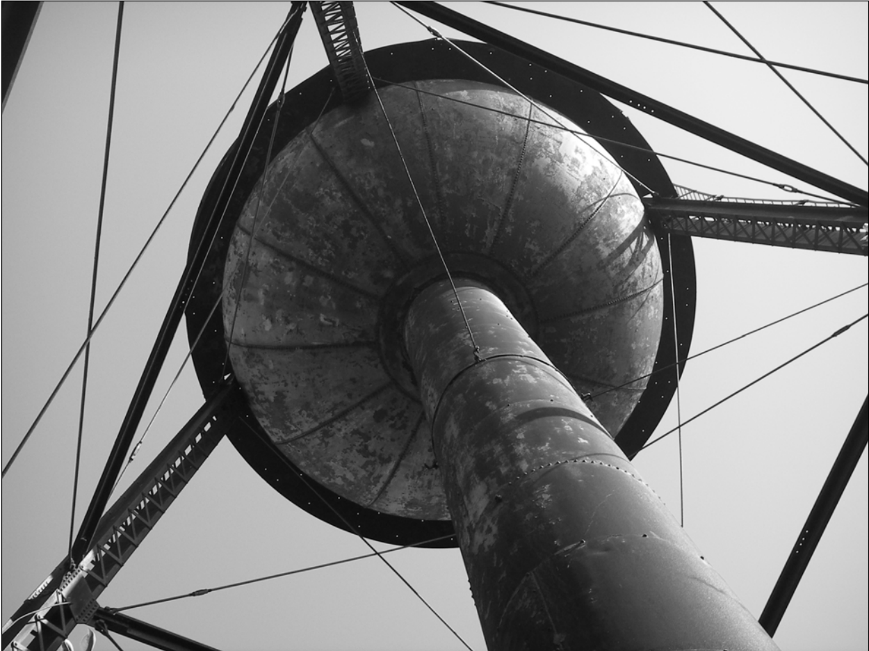
Photo 7. Detail showing the Water Tower's wet riser, tank base, tower legs, and cross-braces.
