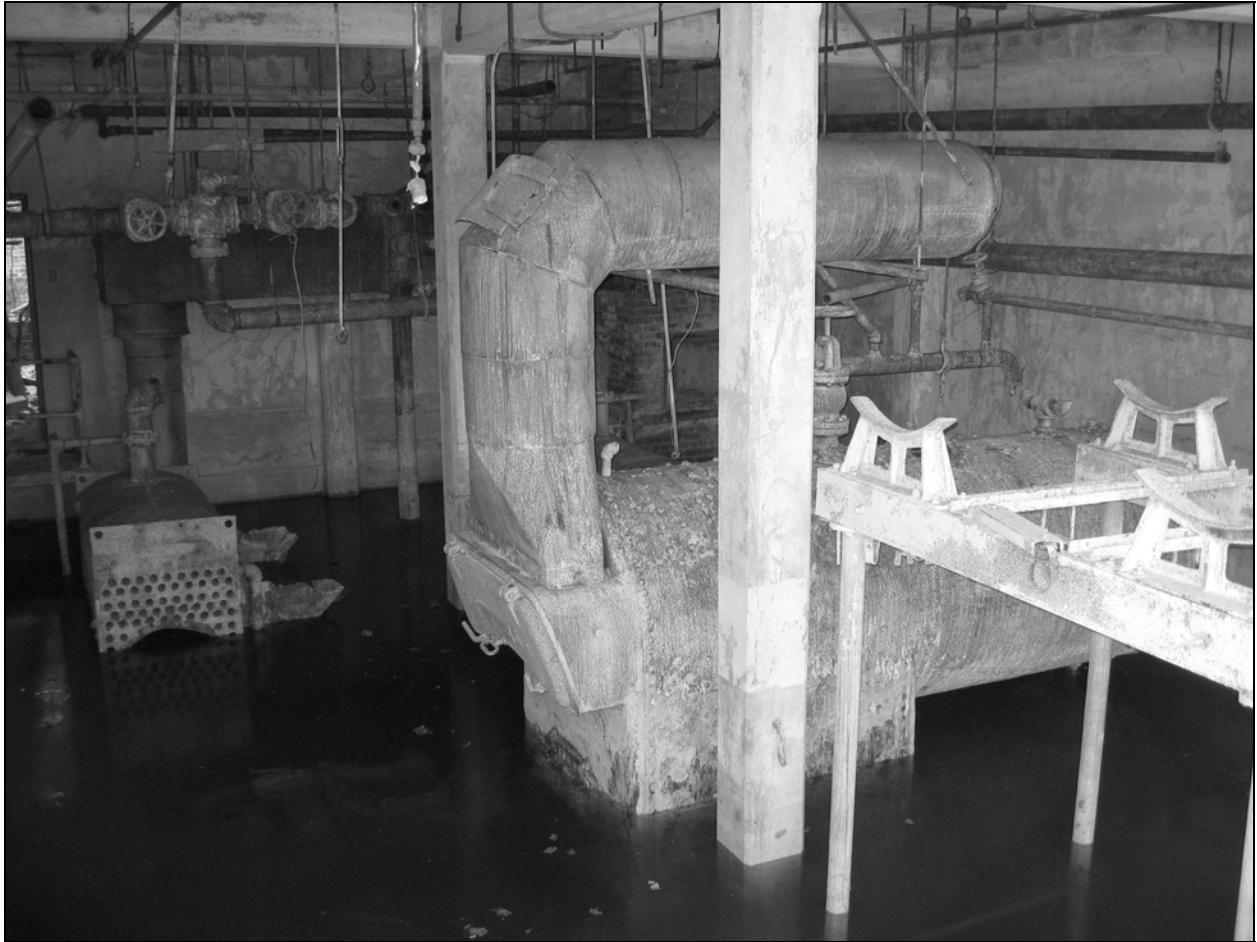
Photo 15. Interior of boiler room-utility area, facing south. Approximately 2 feet of standing water covered the floor when the photograph was taken.
