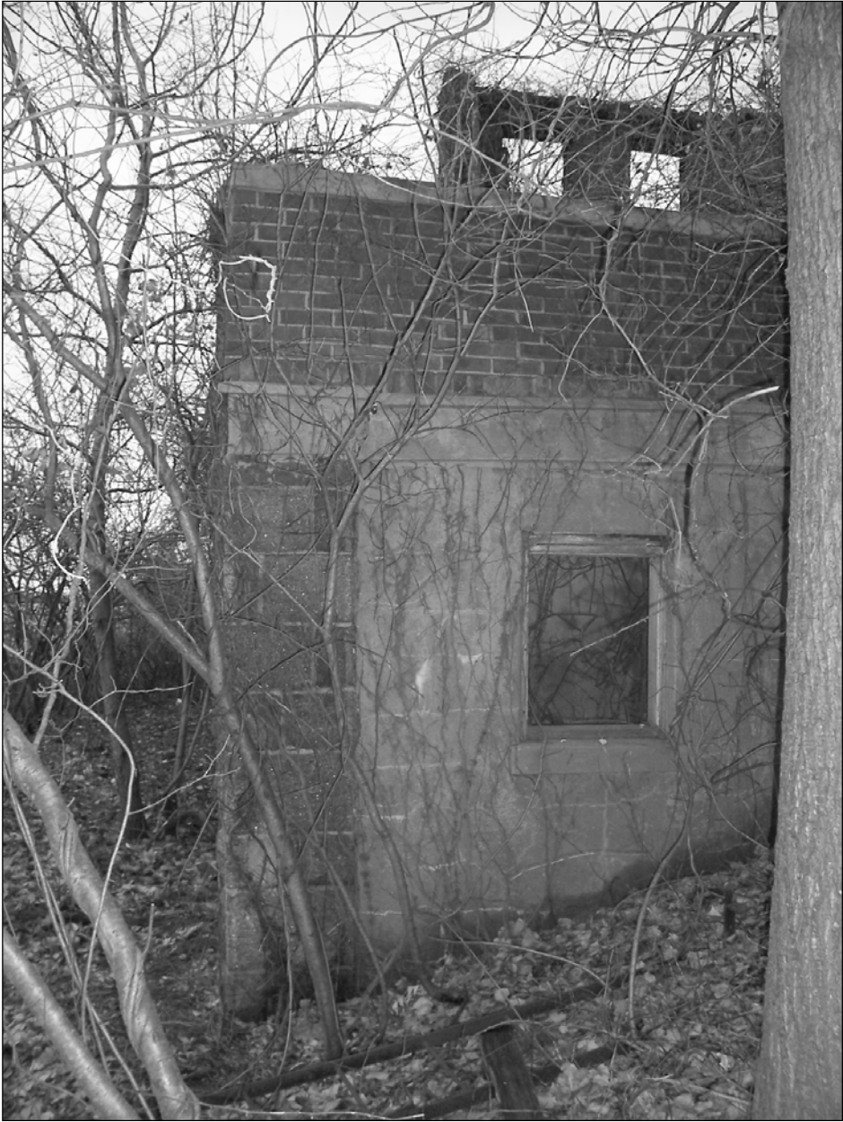
Photo 6. Basement enclosure and rear porch support, detail, north end of western façade, looking east.
