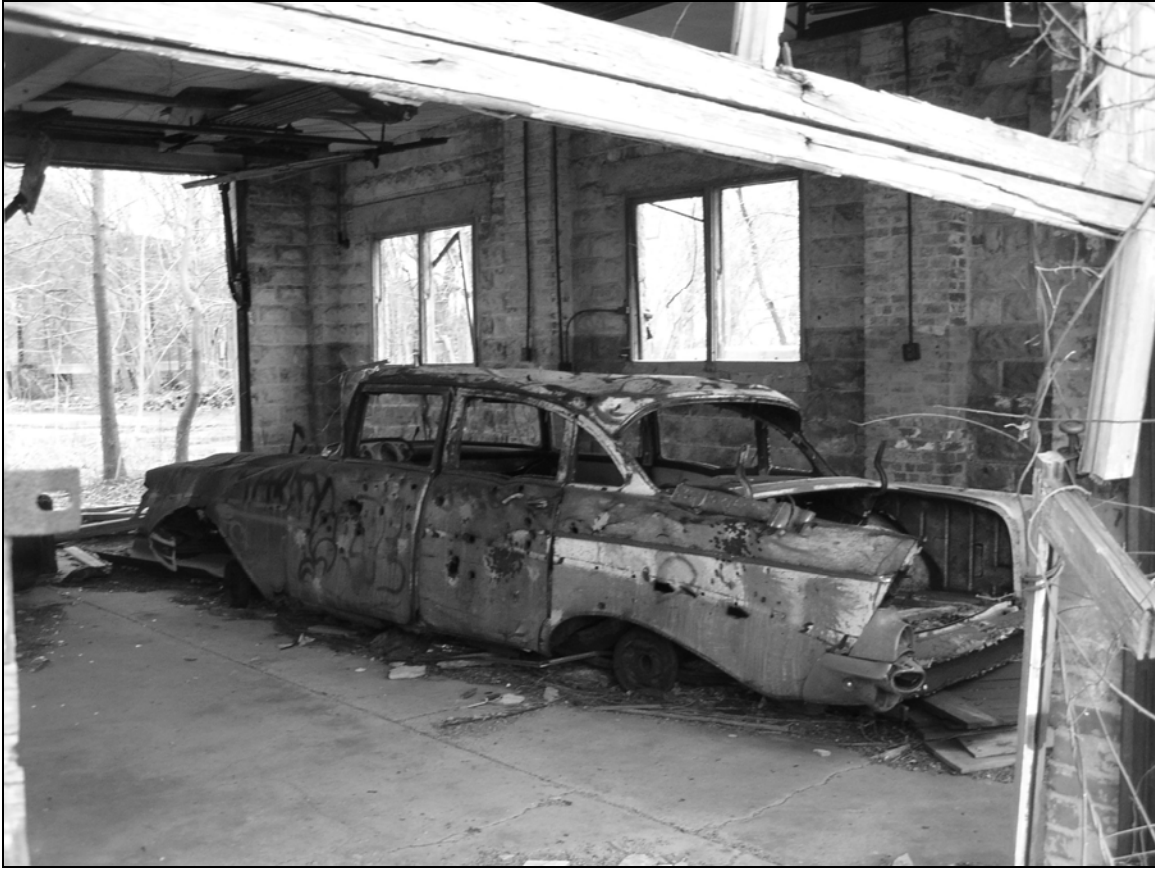
Photo 14. Interior of south vehicle bay of western wing, with abandoned car, facing southeast.
