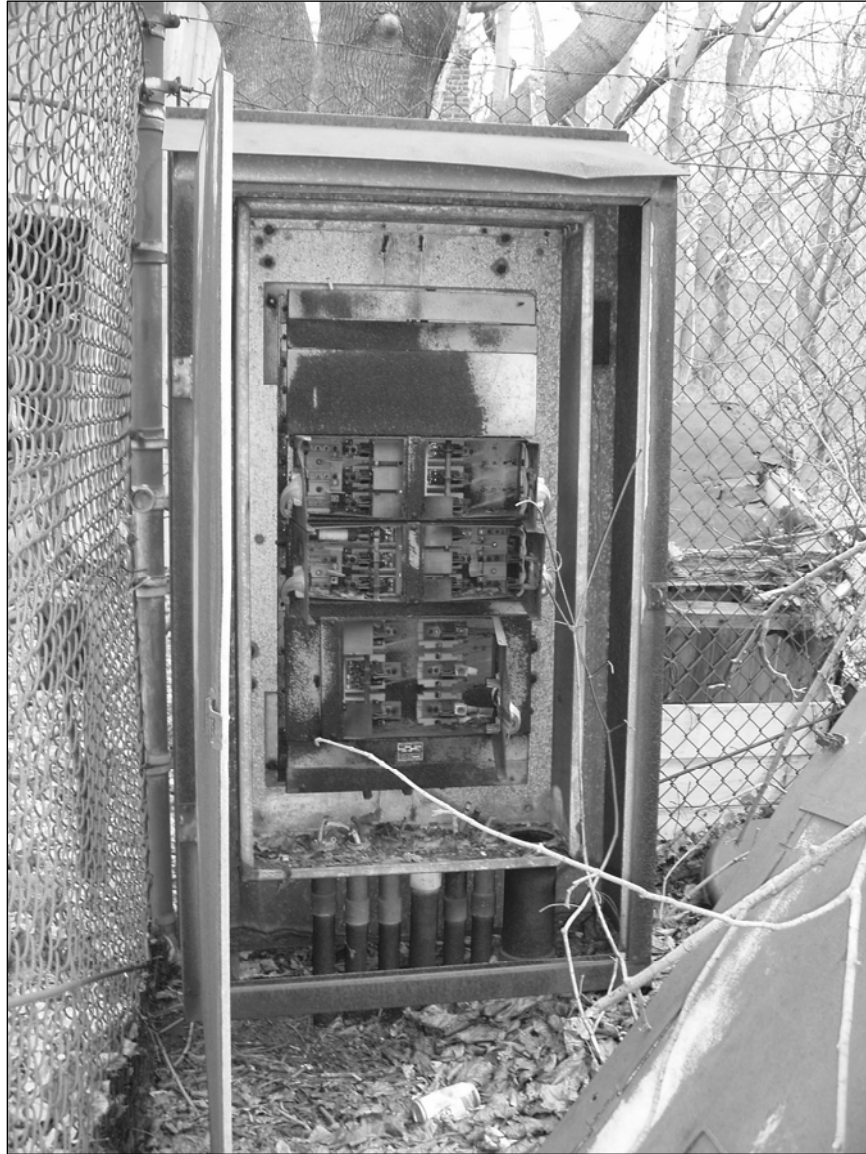
Photo 4. Curcuit breaker cabinet, facing northeast.
