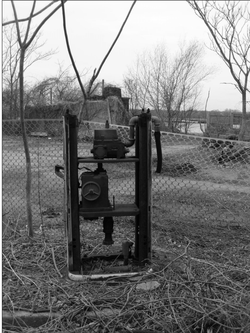
Photo 2. Remains of gasoline fueling pump in concrete island, west of Building 40, facing west.
