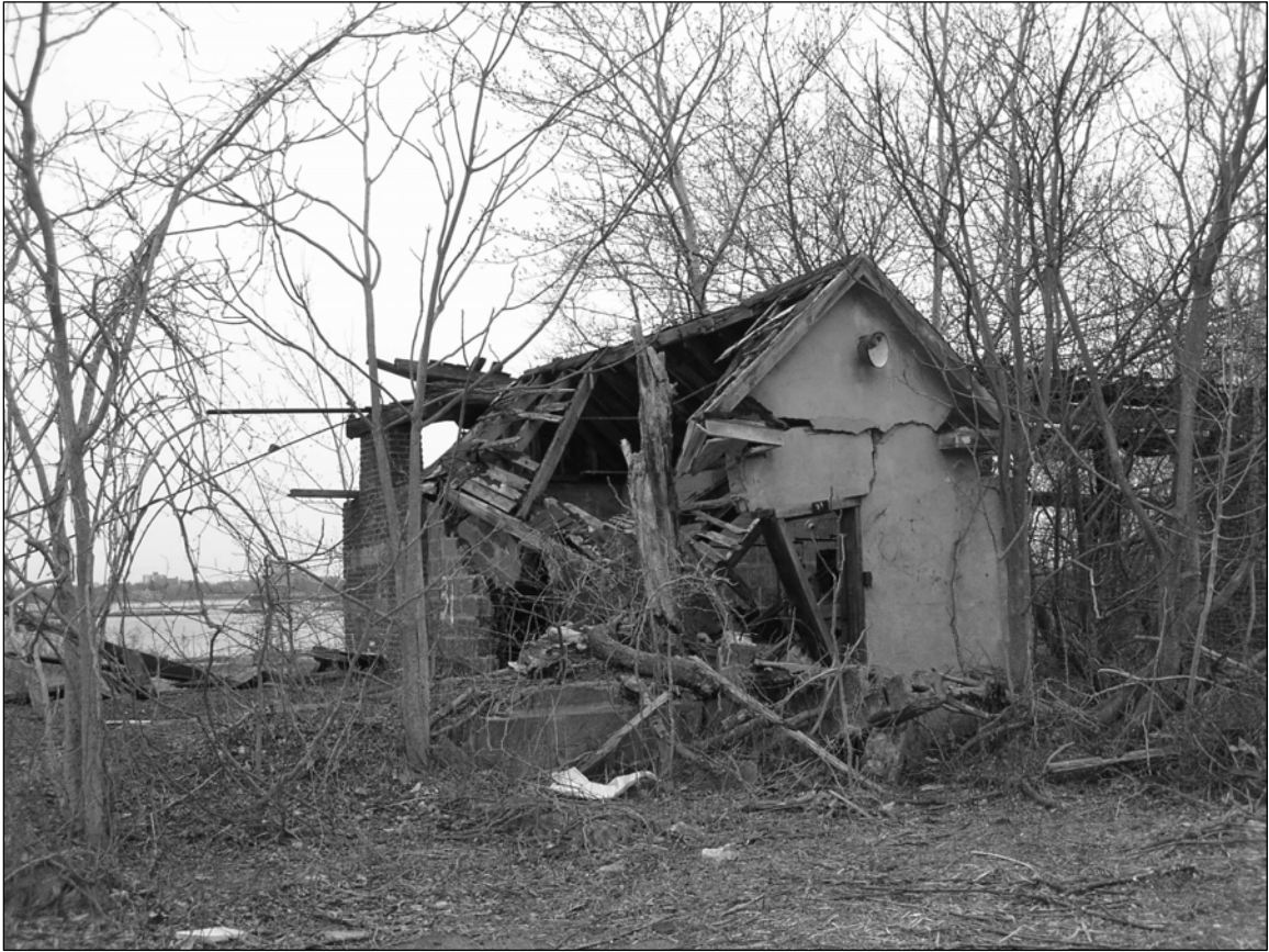
Photo 2. Southeastern façade and collapsed southwestern wall, facing northwest.
