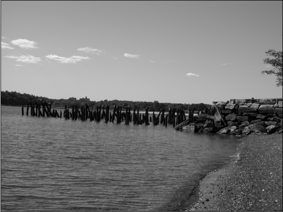
Photo 3. View of southwest side of Passenger Dock and adjacent seawall looking west.
